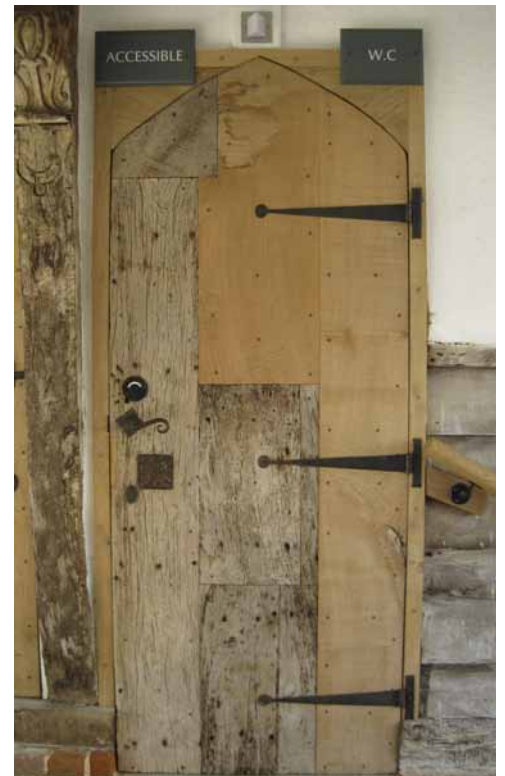
A repaired door at Finchingfield Guildhall clearly showing original and new oak. © David Grech.
