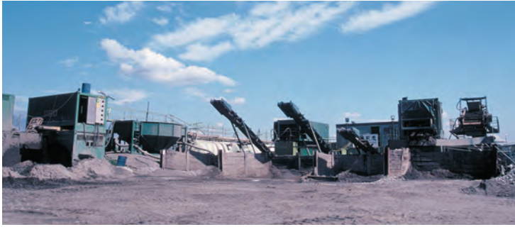
The Royal Arsenal, Woolwich: during the site's regeneration, this was the largest soil-washing plant in Europe. © OA
