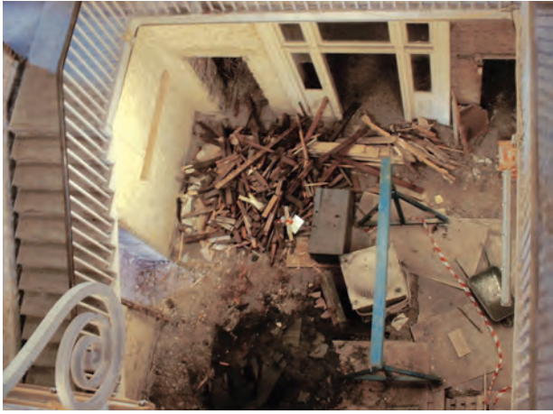
Above: View of the stairwell within Building 37 (Grand Store) ahead of restoration, Royal Arsenal, Woolwich. © BHL
