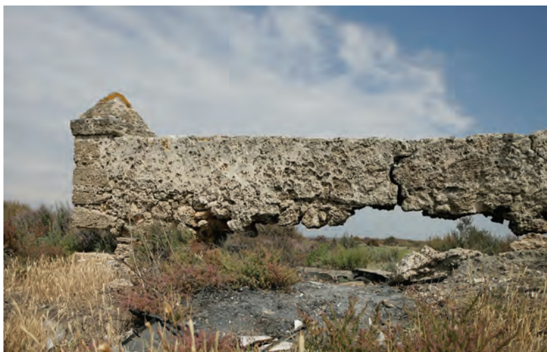
The poor condition of Battery No. 1, Real Carenero, Cadiz, Andalusia. © UCA
