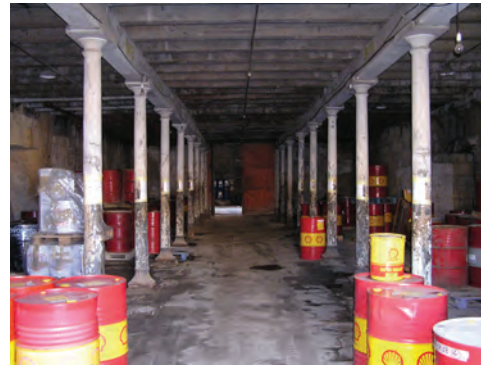
Interior view of an equally large interior space within No. 1 Dock, Grand Harbour, Malta. © EH
