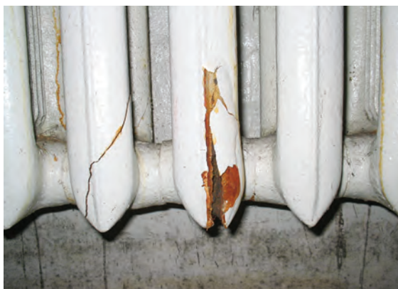
A burst radiator at the Battery, Tallinn, caused by water accumulating in the system over winter when the building was vacant for the first time. © EH
