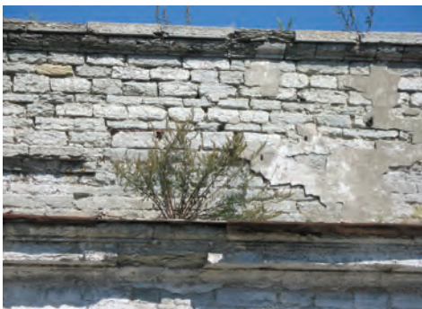
The condition of the stonework at the Battery, Tallinn. © EKA
