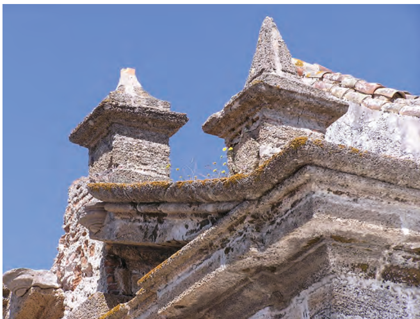
The condition of the central feature of the main range of buildings, Real Carenero, Cadiz, Andalusia. © EH
