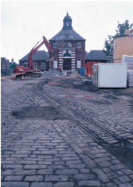
The area in front of the Brass Foundry showing the original cobbled road with inset tracks, Royal Arsenal, Woolwich. © OA
