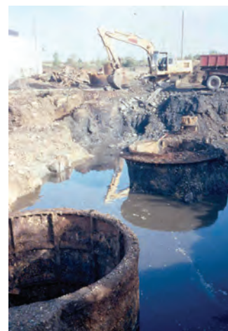
It may be possible to avoid extensive and costly excavation of certain types of contamination. The Royal Arsenal, Woolwich. © EH
