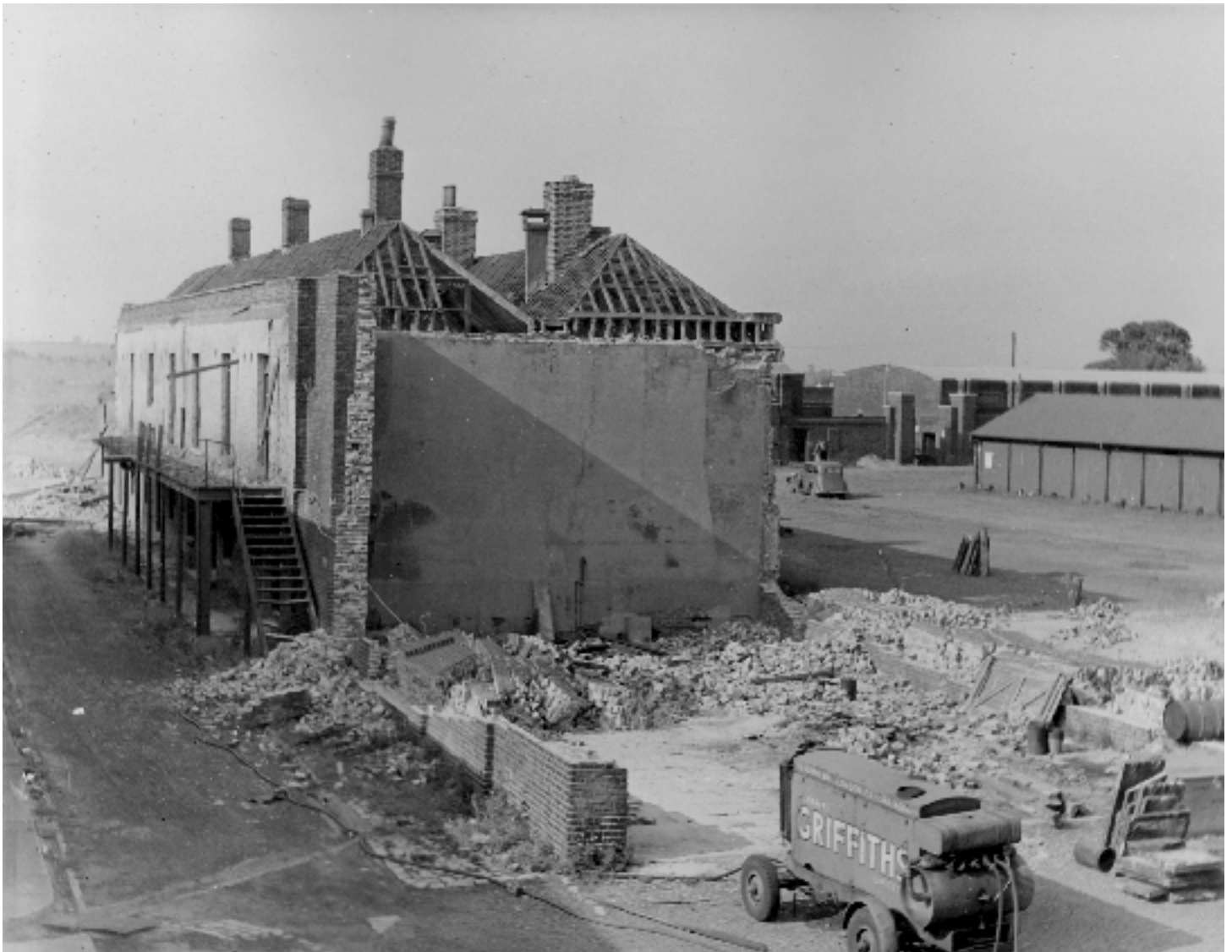
Tilbury in the late 1940's, showing the Soldier's Quarters being demolished, with the Parade Ground occupied with 19th-century waggon sheds
