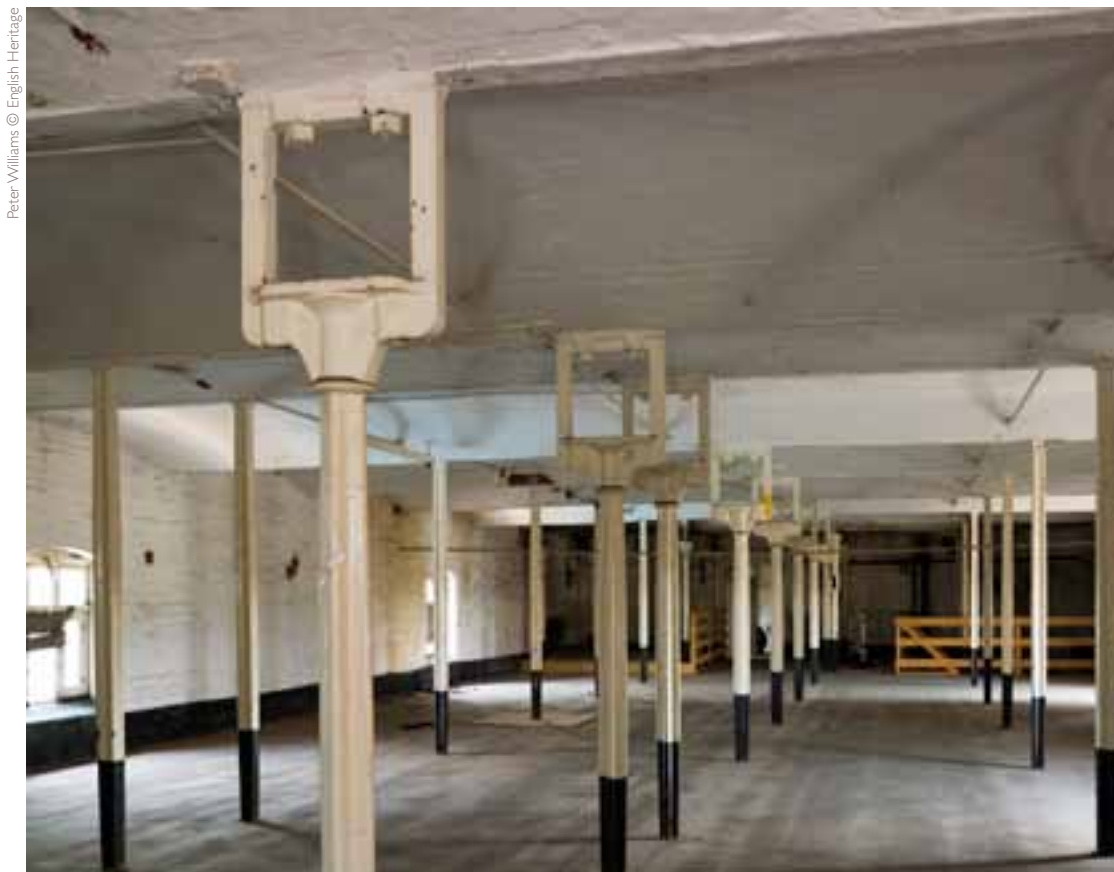
Third storey of the main block, 2001, showing housings for the horizontal main shaft. Proposals for the re-use of the building have necessarily focussed on issues with the iron frame, including problems with the pioneering design and casting defects
