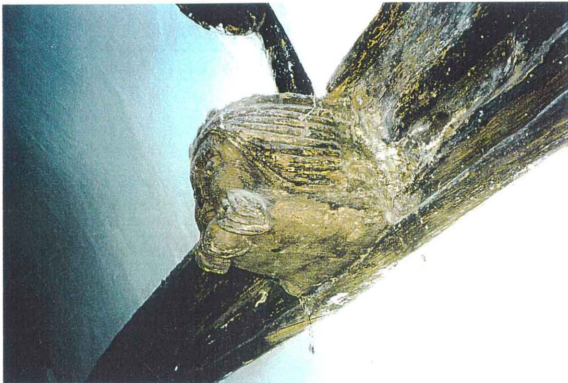
Figure 3: Photograph of stub-tie at T16, north side (Philip Scorer)
