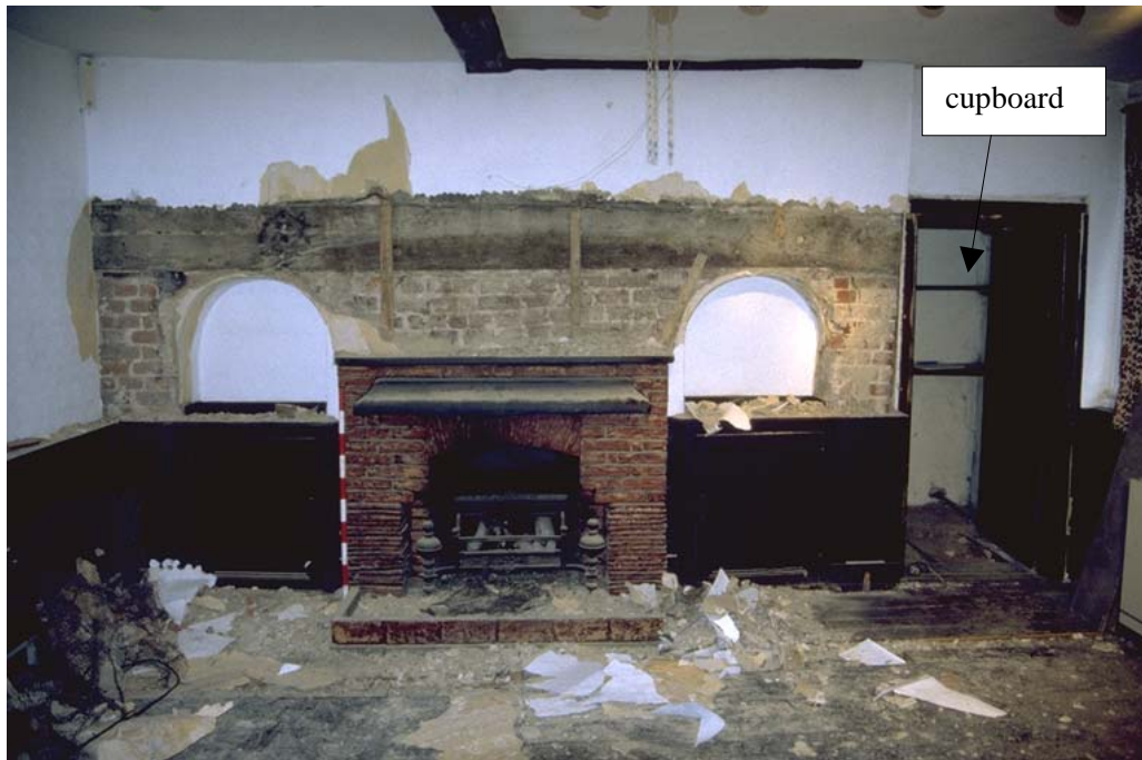
Figure 5: Southern elevation of the Museum (northern face of chimney stack) - 1m scale
