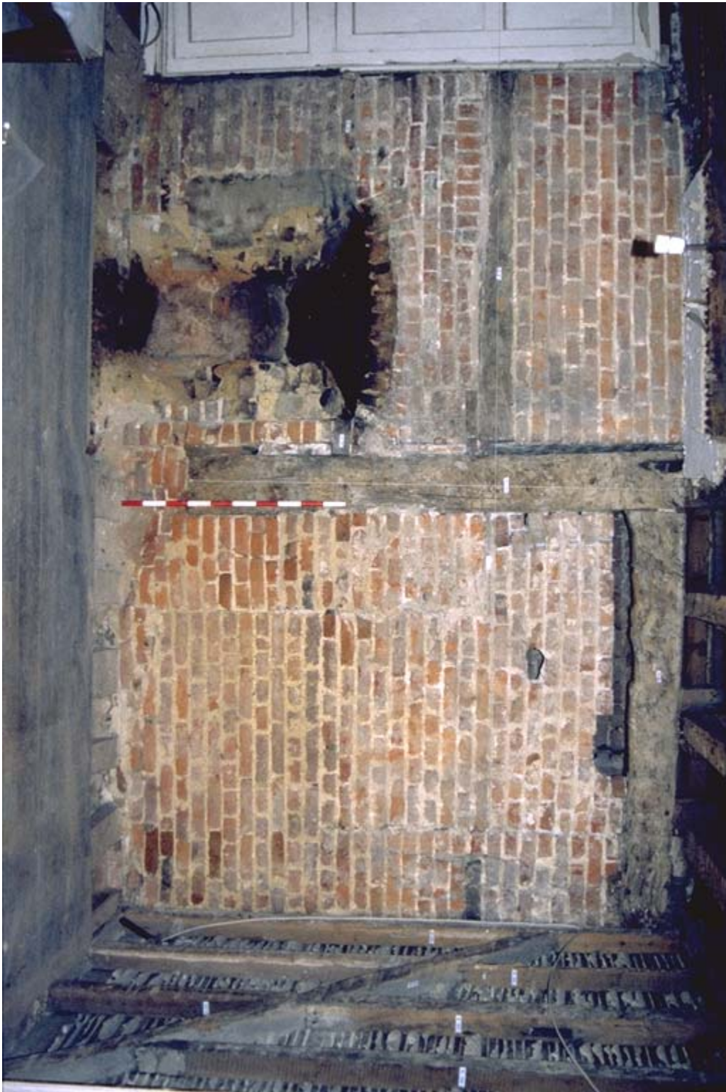
Figure 4: Southern elevation of the western chimney stack prior to investigation works (1m scale)
