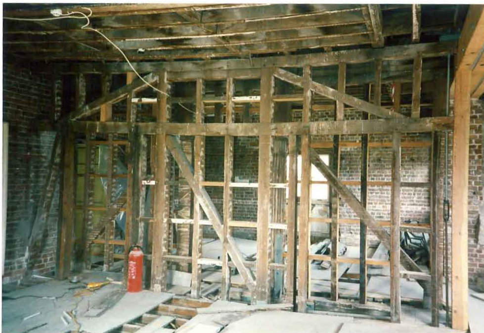
Figure 10: Photograph of south face of partition E, with partition F behind on the bedroom level (C Groves)
