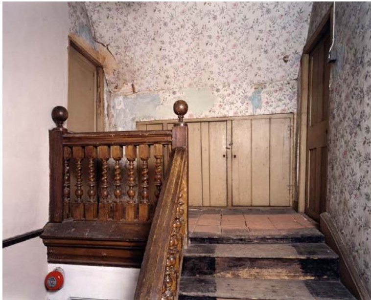
Fig 59. The head of the north stair, from the north. This is the only portion of the two late 17th-century stairs to remain relatively unaltered. (NMR BB032507)
