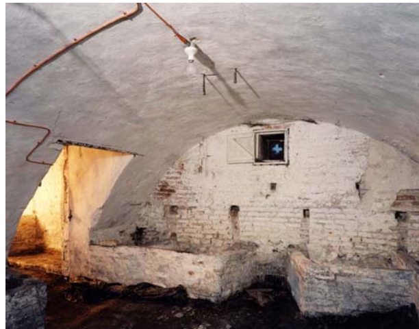
Fig 63. The large transverse cellar room from the south-west, showing the blocked fireplace (?) in the end wall. (NMR BB032446)
