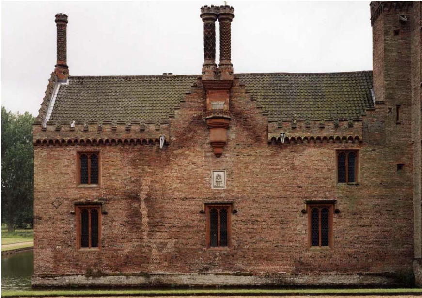
Fig 54. The North range east of the gatehouse: the moatside (north) elevation. (NMR BB032396)
