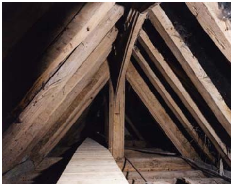
Fig 53. The king-post roof over the west range, seen above the later ceiling at collar level. (NMR BB032498)
