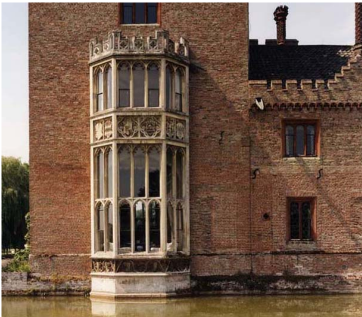
Fig 64. The junction between the south-east tower, as rebuilt in the 19th century, and the remainder of the east range, showing the surviving evidence for 18th-century sash windows to the right of the 19th-century bay window. (NMR BB032399)
