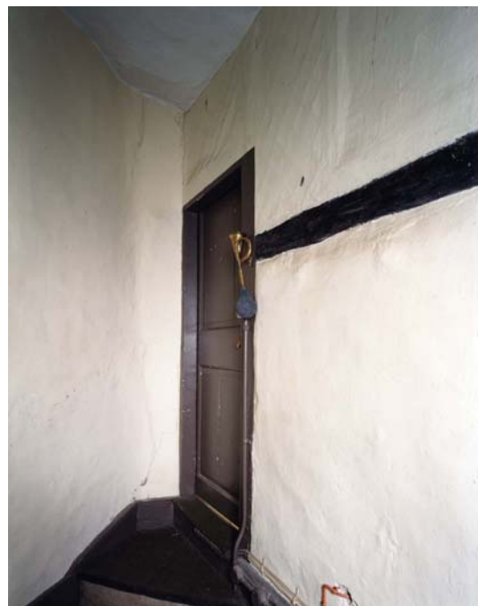
Fig 58. The doorway to the attics east of the gatehouse. Papered over borrowed lights can be seen above and to the right of the door. (NMR BB032445)
