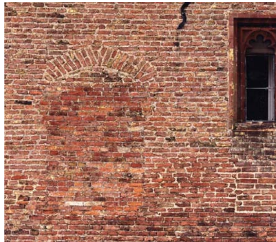
Fig 15. A blocked original window on the moatside elevation of the east range. (NMR AA026767)
