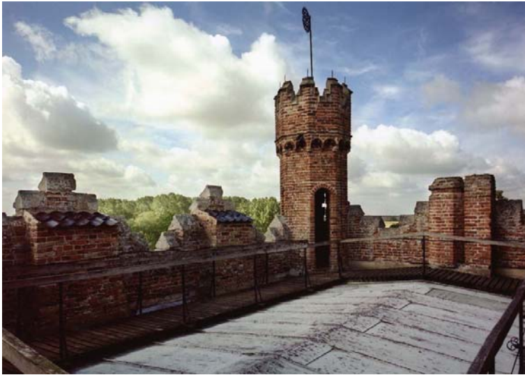
Fig 44. The gatehouse rooftop from the north-east. The stacks serving the King's and Queen's Rooms are to the left, capped with pantiles. (NMR AA026770)
