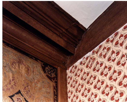
Fig 60. The late 17th-century cornice on the first floor of the north range west of the gatehouse. The Gothic wallpaper dates from Buckler's 19th-century work. (NMR BB032506)
