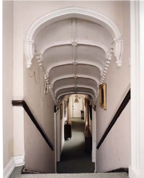
Fig 104. The first-floor passage along the courtyard side of the west range, seen from the higher floor level of the Saloon block. (NMR 032492)
