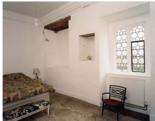
Fig 50. The larger of the two recesses is a blocked window, exposed in 2001. (NMR BB032457)
