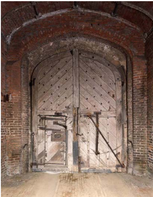
Fig 25. The double gates (and wicket gate) barring the entrance to the courtyard. (NMR BB032415)
