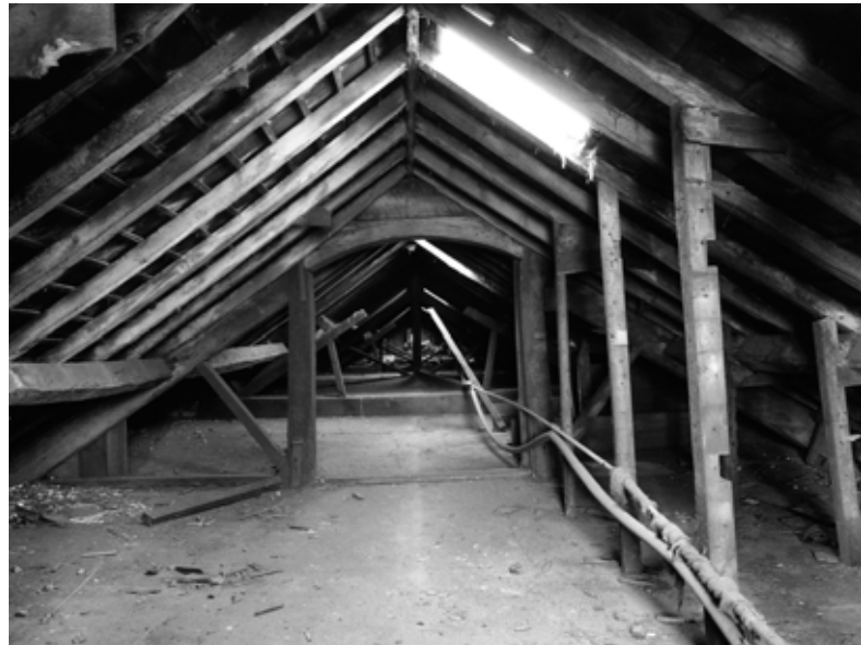
Fig 30. The attic and original roof structure of the east extension, from the east.
