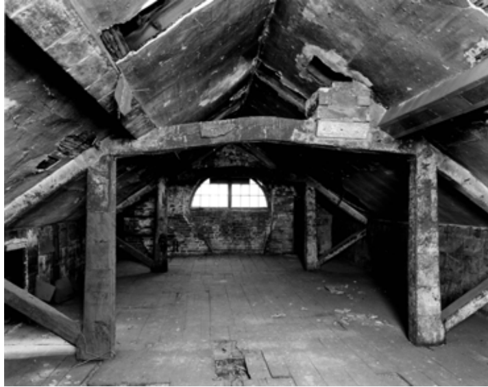
Fig 19. The attic and queen-post roof of Long Mill, from the north. One of the flues inserted in the 1790s to serve the school-room stoves, remains on top of the right-hand end of the collar. (BB001912) See also the cross-section, Drawing 3.
