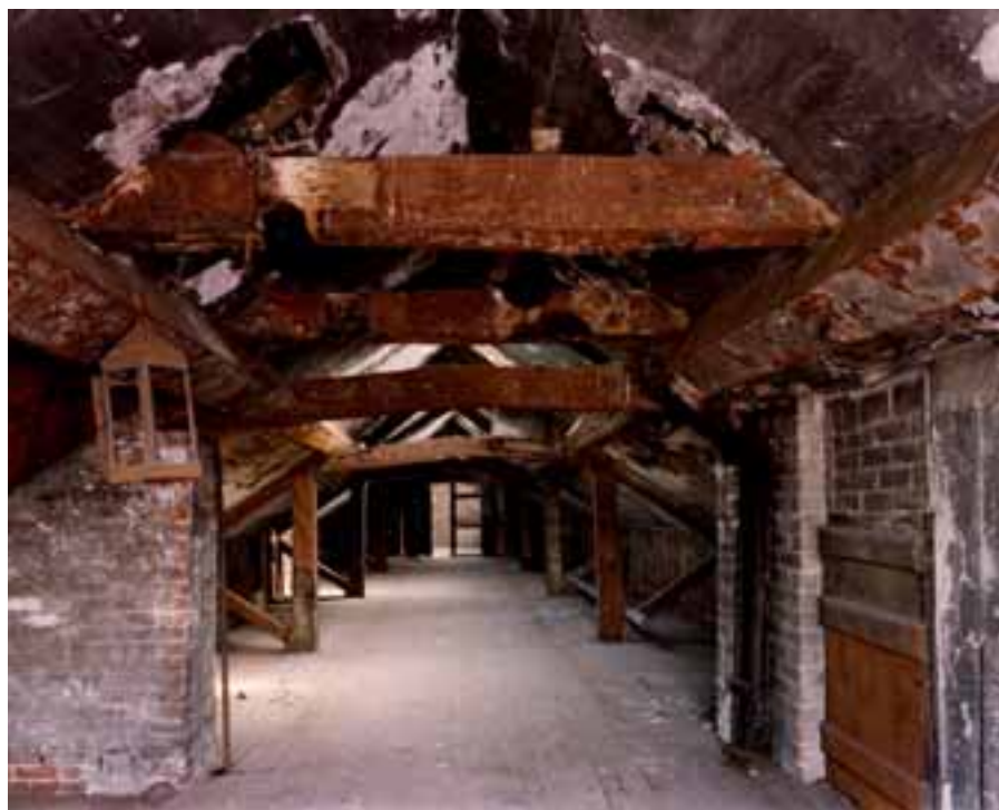
Fig 20. The attic of Long Mill, seen from the north. The metal plates sheathing the truss timbers and other exposed timbers are clearly seen. The two bearers suspended above the purlins in the foreground supported the former cupola housing the mill clock and bell. Traces of line-shafting are also visible. (BB001911)
