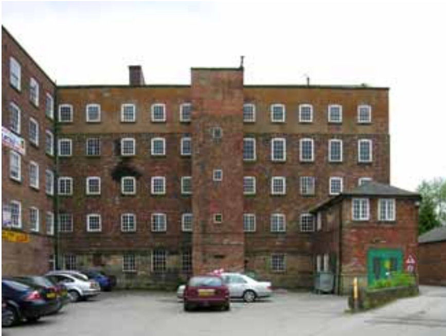
Fig 14. The east elevation of Long Mill, with Middle Mill at right-angles to the left. The leat passed directly alongside the stone ground floor. The stone ground floor and rendered brick fourth floor are clearly differentiated.
