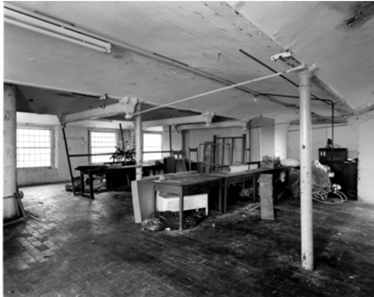
Fig 42. Interior of the east-west arm of West Mill from the south-west, with the stair compartment showing to the left. The columns, the beams they support and the brick vaults are original features, but the transverse tensioning beneath the vaults is later. (BB001919)
