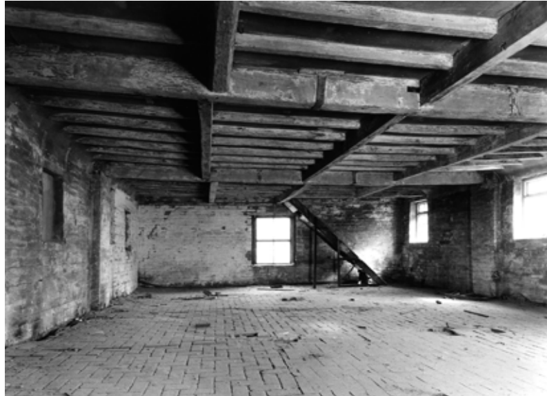
Fig 29. The first floor of the east extension from the west, showing the brick-paved floor and grid of ceiling beams. The makeshift ladder stair at the far end occupies an original stair position.
