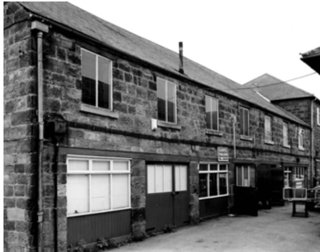
Fig 60. The eastern addition from the north, showing the formerly open-fronted ground floor. (BB001883)
