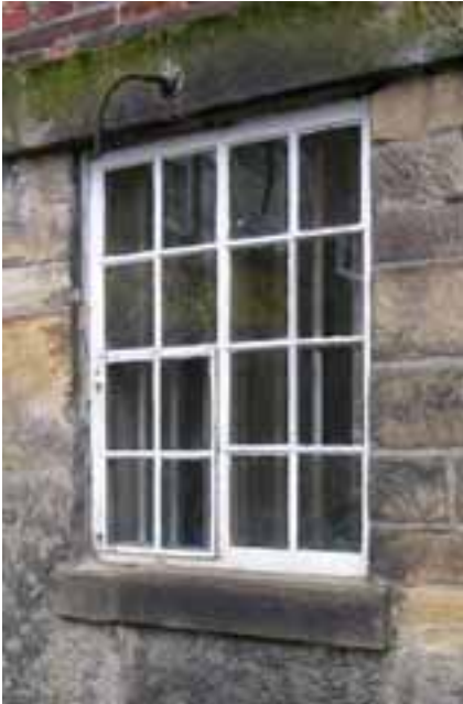
Fig 18. One of the early timber and iron-casement windows on the east elevation of Long Mill.
