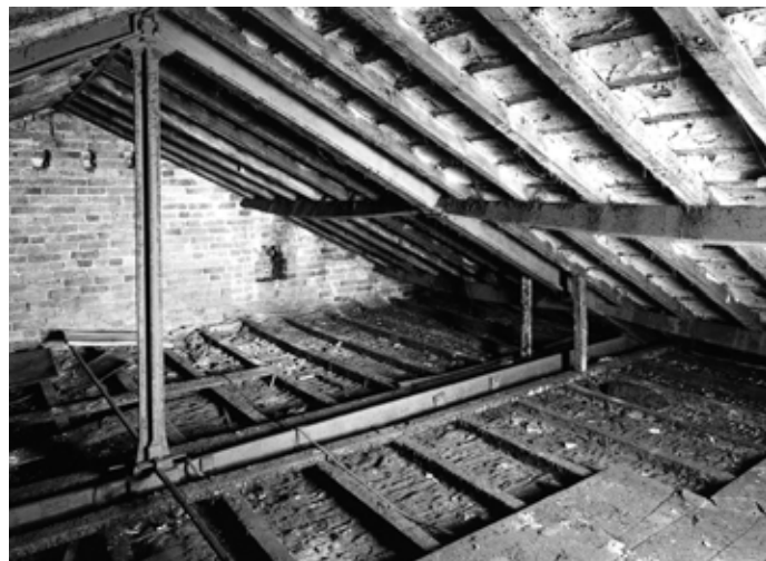
Fig 34 (top). Fireproof brick vaults on the second floor of East Mill, showing cut-outs for a central axial overhead line-shaft.
