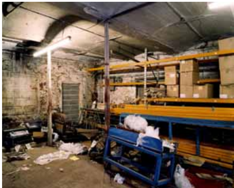
Fig 28. The proto-fireproof ground-floor ceiling of the eastern extension, showing brick vaults springing from timber beams supported on cast-iron columns. (AA051582)
