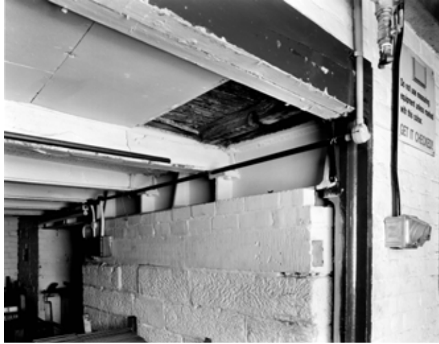
Fig 51. The space beneath the raised ground floor of the north extension. (BB001927)
