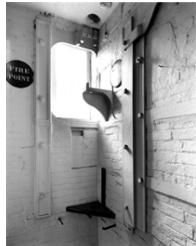
Fig 53. One of the bearing boxes indicating an upright shaft position in the stair well at the western end of North Mill. (BB001930)
