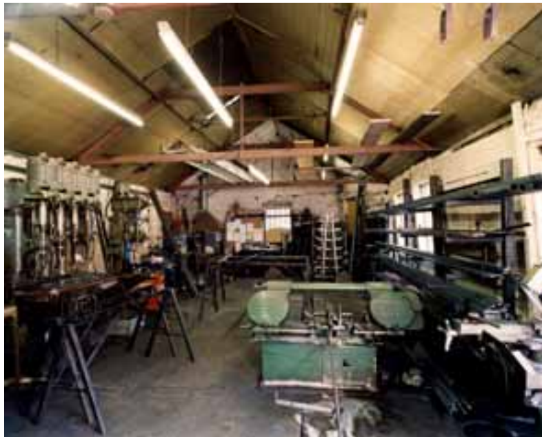
Fig 66. Interior of the Fire Station from the south, showing the cast and wrought-iron tie-beam and collar trusses. (AA051584)
