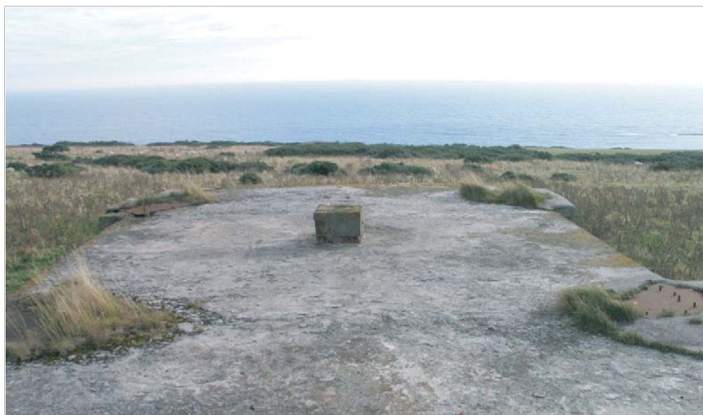
Figure 11 The roof of the TxRx Block, looking east, with the metal footing- plates for the roof- mounted gantry
