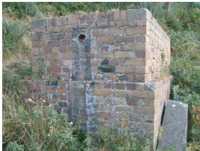
Figure 20 Settling tank forming part of the drainage system from the ablutions block
