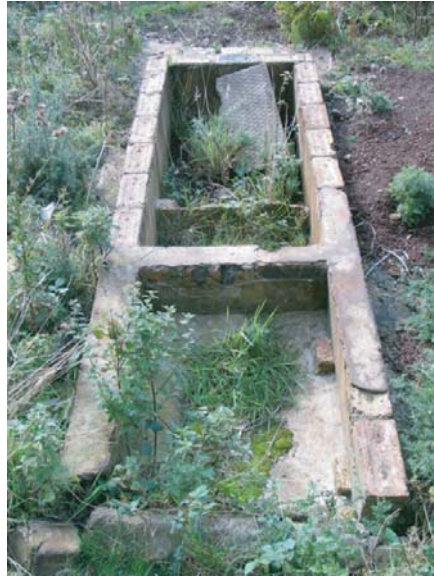
Figure 19 A 'fat trap', part of the drainage system associated with the ablutions block
