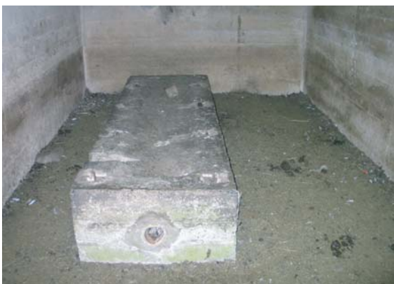
Figure 15 The machine bed, which supported the generator in the Standby Set House
