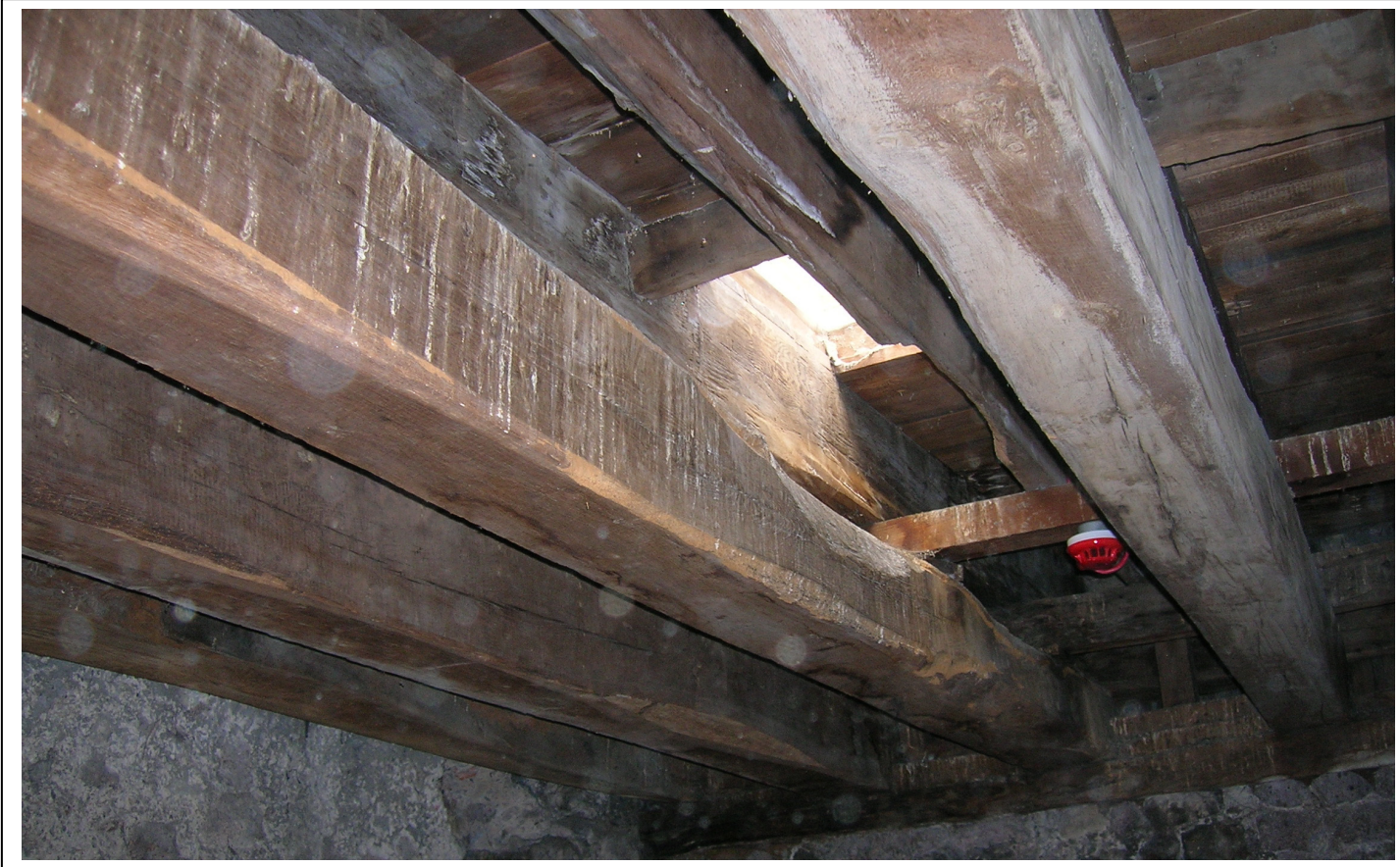
Figure 3: View of the roof timbers of the Chapel of St John the Baptist
