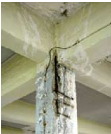
Figure 74 Concrete spalling in Trafalgar House (DP040040)
