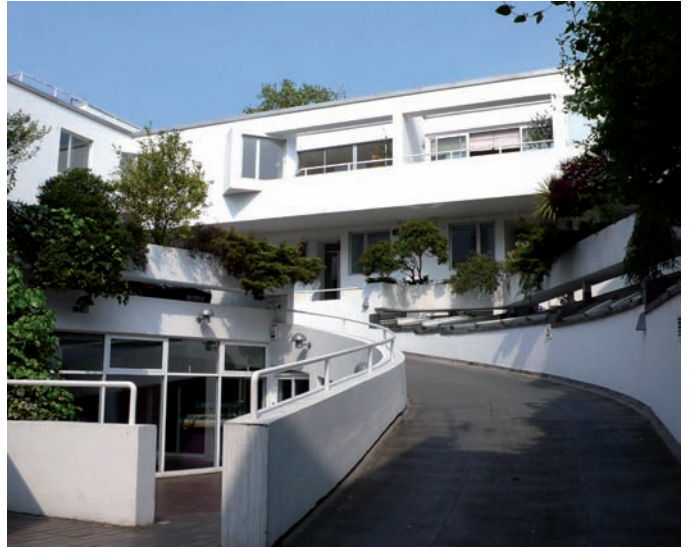
Fig. 1: View looking east, showing renewed (left) and inserted (right, under ramp) office fenestration (DP040021)
