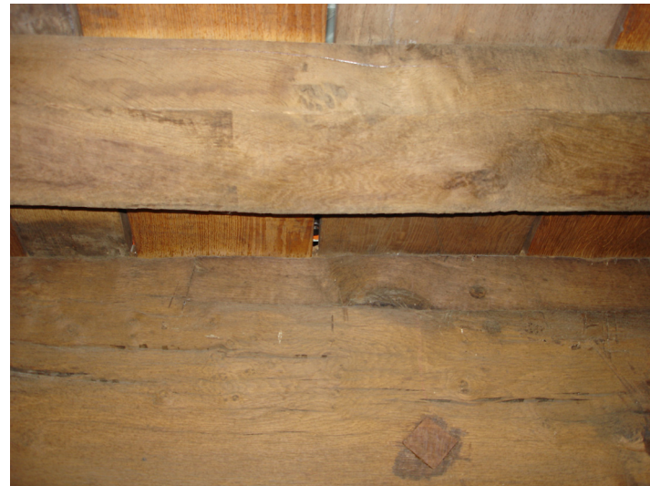
Undersquinted abutment of furring pieces on tiebeam
