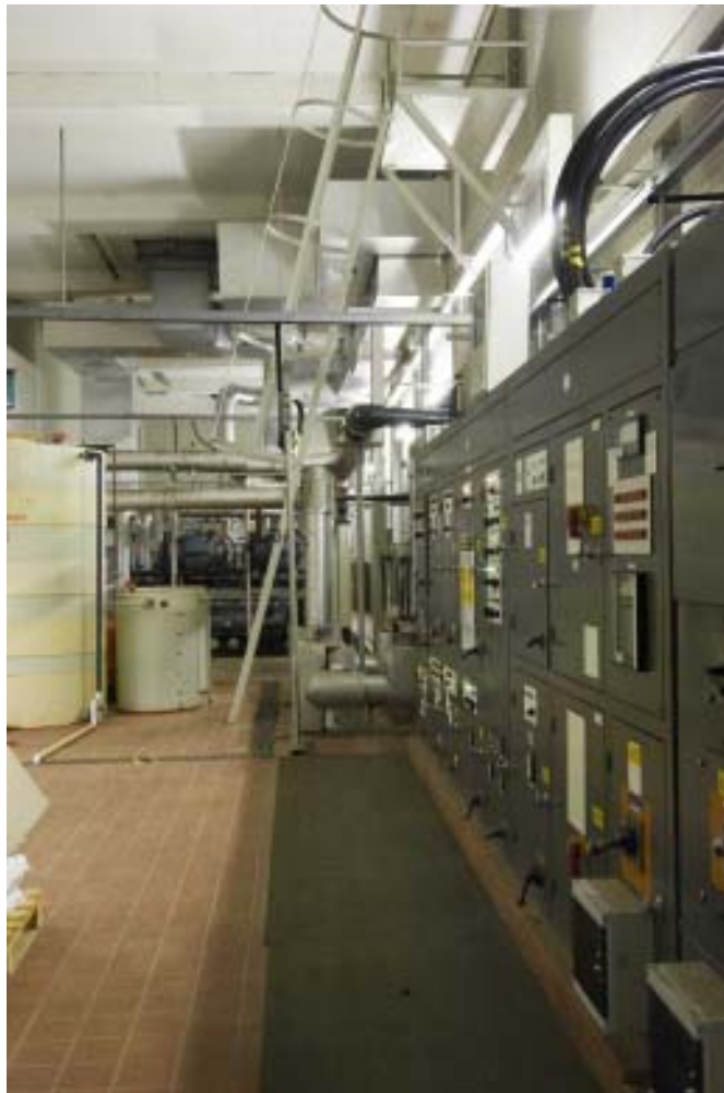
Figure 167 Building 349, Jaguar Flight Simulator, part of the cooling plant that was initially required to cool the heat generated by the lights over the large terrain model. (c) English Heritage DP027203
