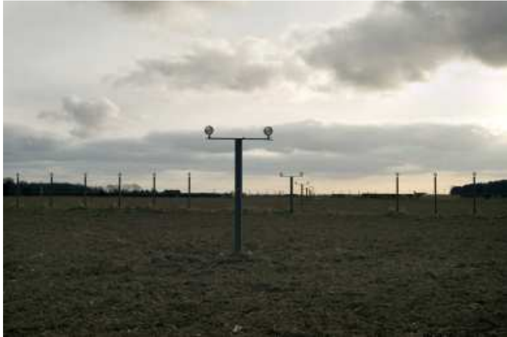
Figure 5 Runway approach lighting to northeast of runway off Scottow Road. (c) English Heritage DP029257
