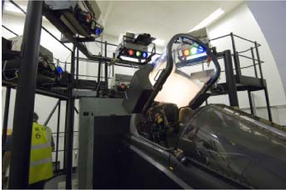
Figure 174 Jaguar Flight Simulator building, training cockpit and to the rear the projectors used to project the moving images on to the hemisphere. (c) English Heritage DP027194
