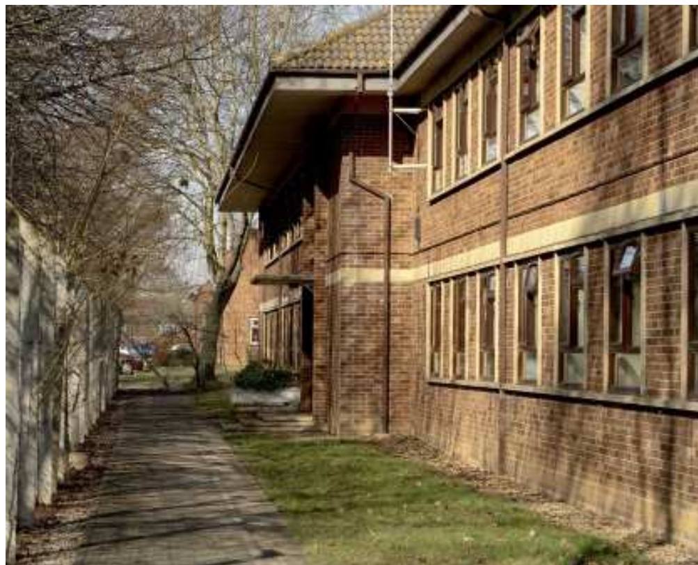
Figure 75 Salmon block, Building 202A, to the north west of the Airmens' Institute, is a relatively unusual example of a permanent 1950s barracks buildings. It too originally had a flat roof that has been replaced with a gable roof. (c) English Heritage AA0544460
