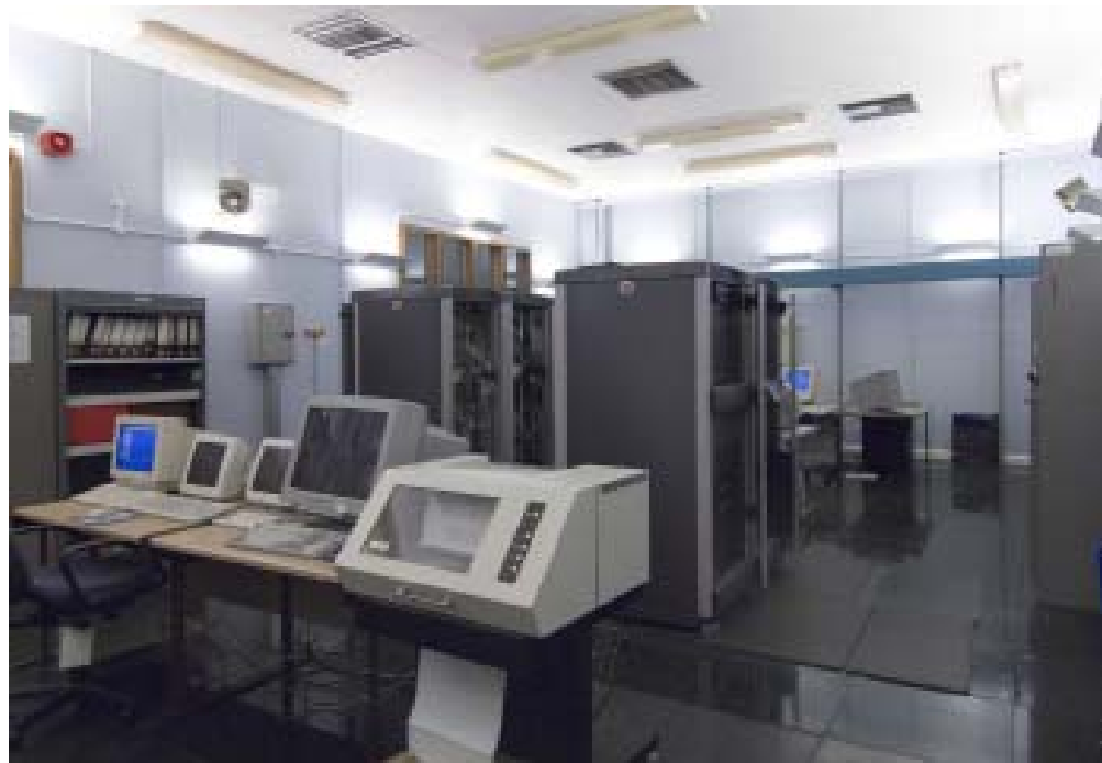
Figure 171 Jaguar Flight Simulator building, main frame computer used to mimic the aircrafts operating systems and to project images of changing terrain on to hemisphere in front of the simulator. (c) English Heritage DP027200
