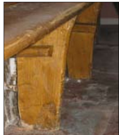
Fig. 55 Detail of the bench supports, similar to those sometimes used for church pews. [DP047062]
