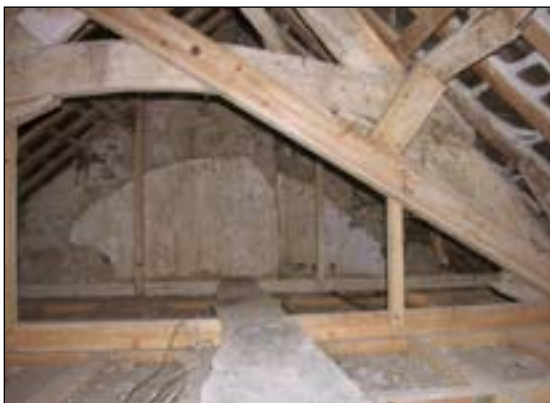
Fig. 24... View into the roof space above the parlour, showing a roof truss with the curved collar and the plaster scar of the barrel vault over the northern chamber. [DP047052]
