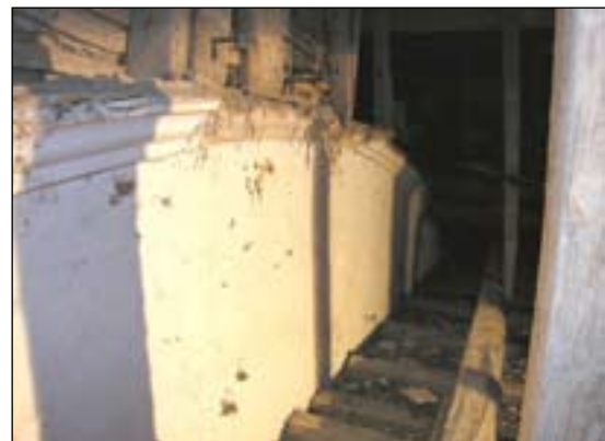
Fig. 25 View into the roof space above the parlour, showing the plaster scar of the barrel vault over the present bathroom. [DP047053]
