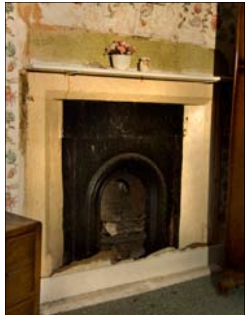
Fig. 36 The granite fireplace of the upper chamber in the southernmost room of the north-west extension. [DP031671]
