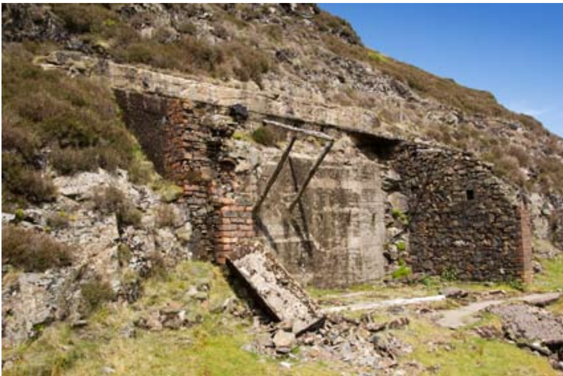
Figure 11. View from the south of the hand-sorting shed. © English Heritage 2007, NMR reference DP054874.
