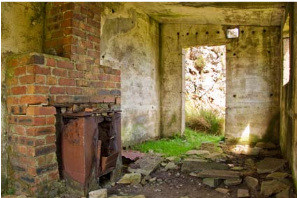
Figure 20. View from the west of the interior of the probable office. © English Heritage 2007, NMR reference DP054881.
