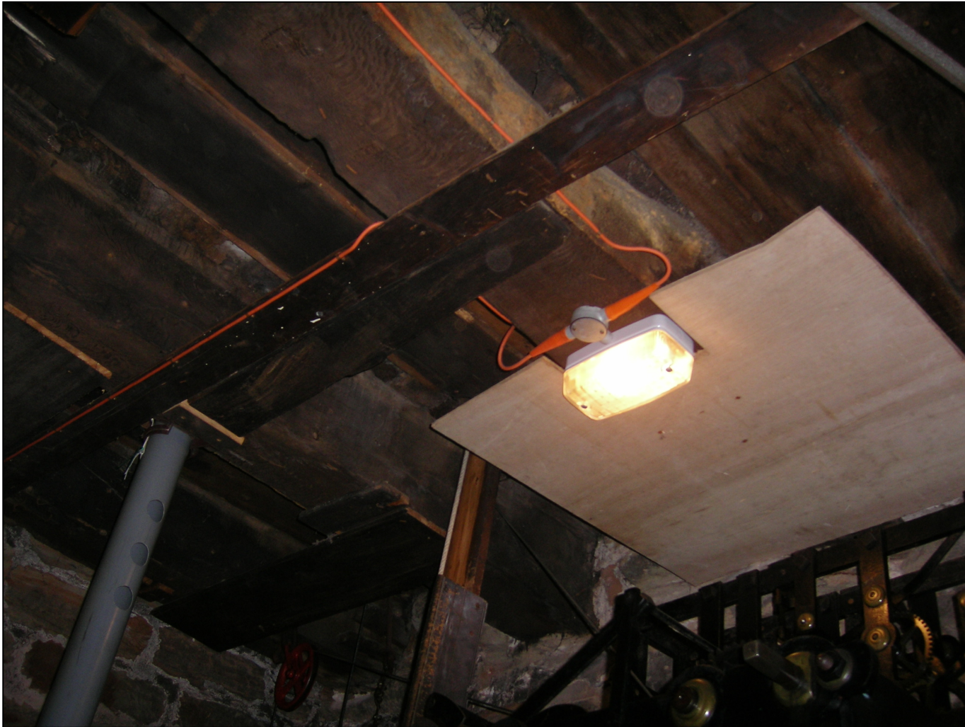
Figure 6: St Swithun's Church, belfry floor, beam 4 to the far left (as viewed from below)
