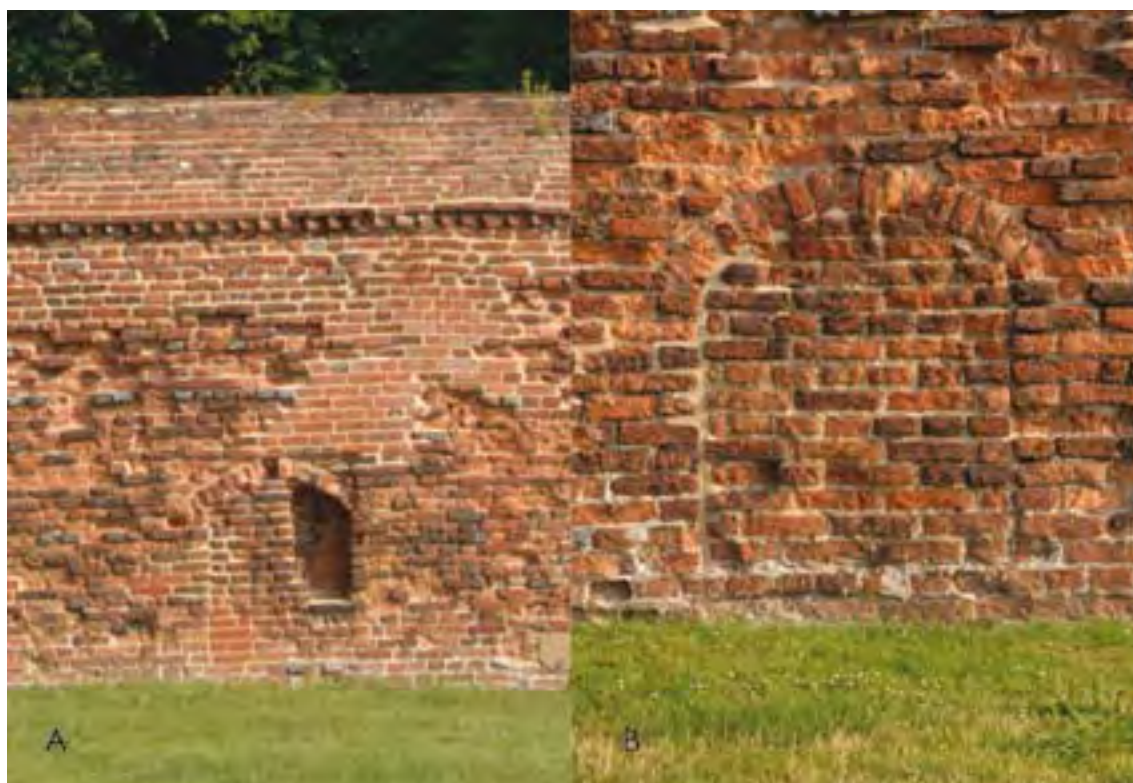
Figure 24: A - Section of the northern boundary wall showing one of the partially blocked bee boles, the dog-tooth string course and the ornamental coping. B - Detail of blocked bee bole.
