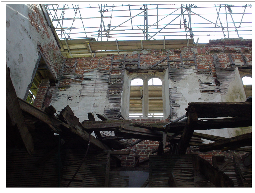
Figure 4a/b: Photographs to show derelict and dangerous nature of the building before room clearance and stabilisation (photos by Peter Rumley consulting archaeologist)
