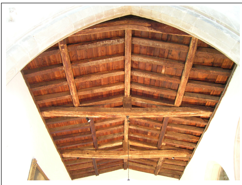
Figure 4a (top): View of the chancel roof looking west to east showing the straight tiebeams of trusses 2 and 3
