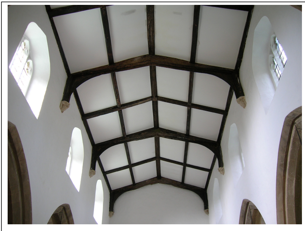
Figure 3a (top): View of the nave roof from the east end looking west
