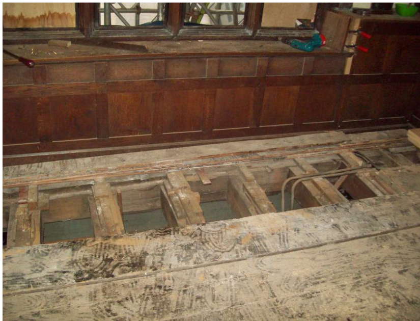
Figure 6a/b: View of the exposed joists to second (top) and first-floor frames (bottom)(viewed looking east to west)
