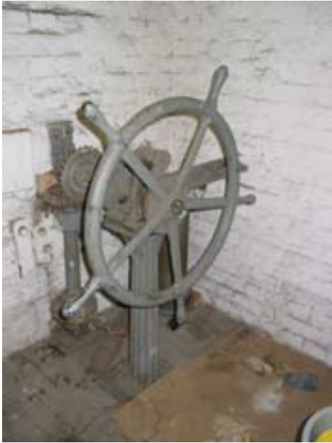
Figure 25: Building 5 (south wing). Wheel house interior: detail showing control wheel for sluice gate (DP098882).
