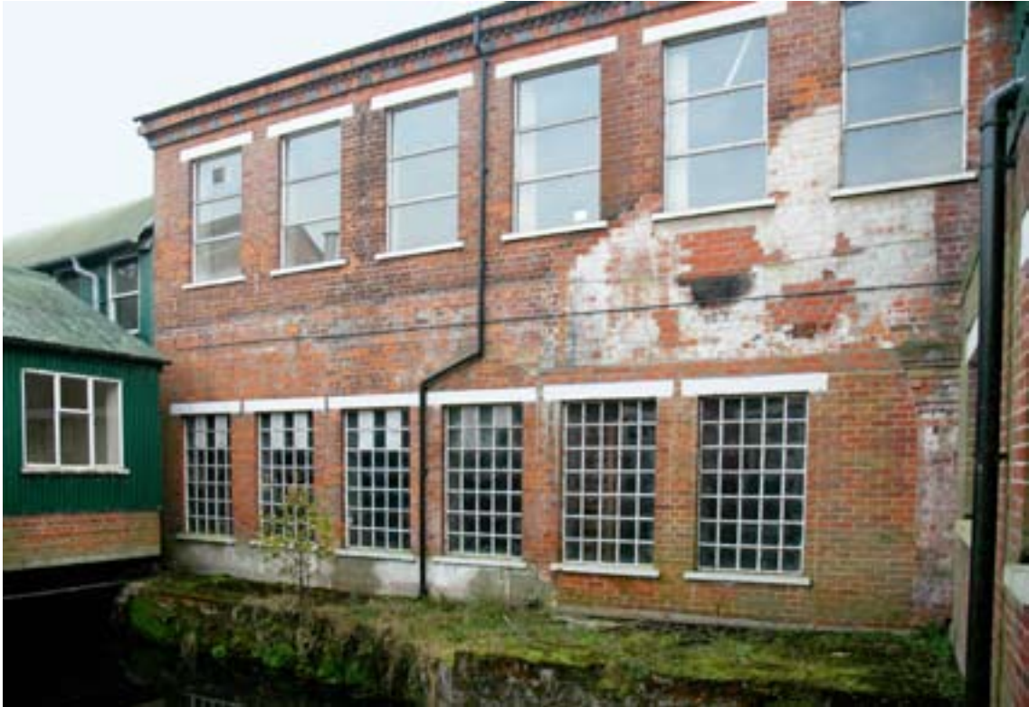
Figure 48 (left): Building 2, north elevation. The ground floor was the salle (photograph: Jon Clarke; DP098889).
