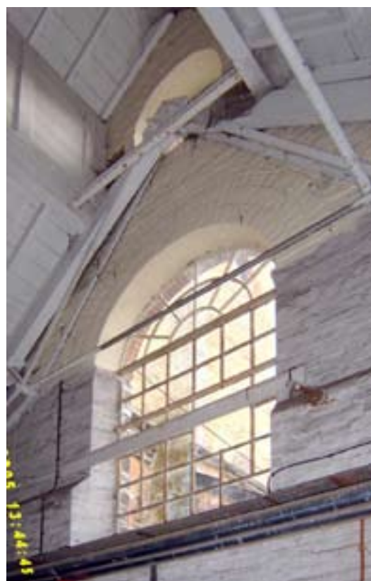
Figure 33: c.1854 element of Building 9, south internal elevation. Note the Polonceau trusses (photograph: Andrew Barber, B&DBC).
