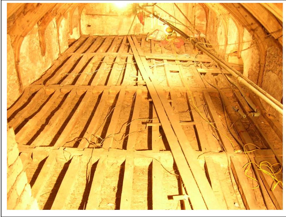
Figure 8 The frame inserted to ceil the great chamber and form the attic floor
