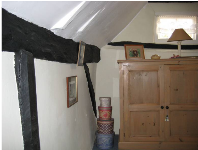
Figure 4: Bay 2 first-floor north wall plate and brace and cross-frame 3 tiebeam, viewed looking north-east
