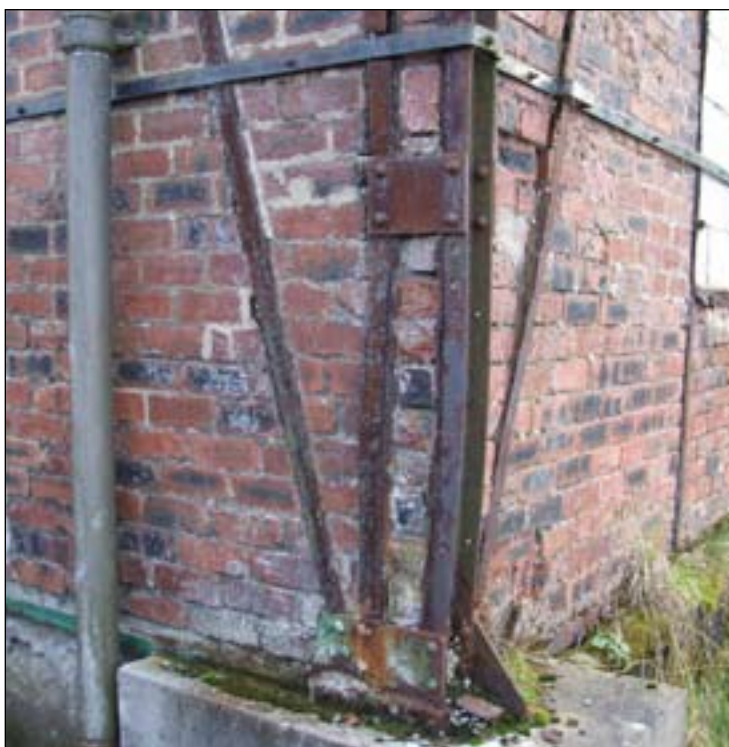
Fig. 14: Steel framing with brick infill, found on the former Gravity Mill constructed in 1908, now Wright Brothers' bus garage, Nenthead. [DPI35362]
