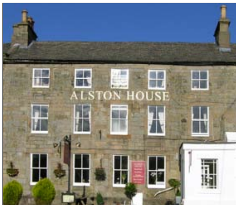
Fig. 11: Rare ashlar masonry on the central part of the mid-18th century Alston House, Townfoot, Alston. [DPI35360]
