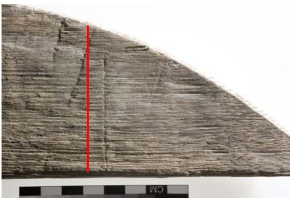
Fig 19: Illustration of where cross section analysis (Fig 20) through timber was carried out
