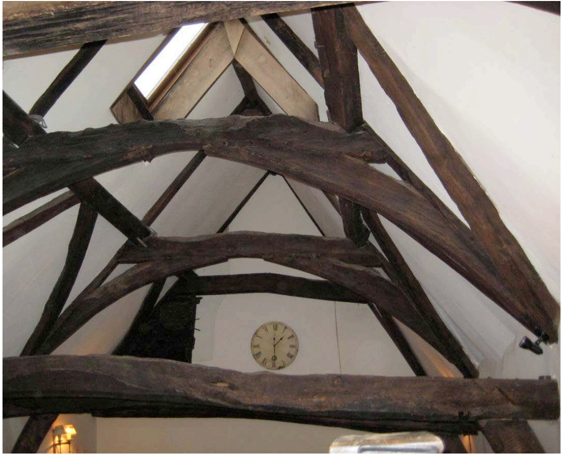
Figure 4: The interior of the open-hall roof in 11 Silver Street, viewed looking south
