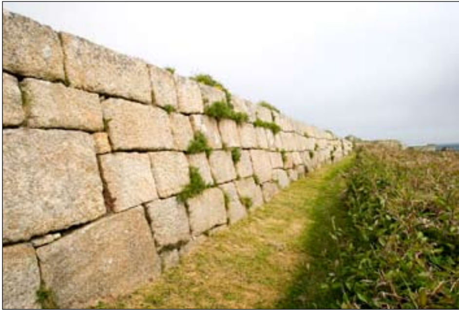
Figure 28. Joint to the west of Redan B – on left of photo [DP022600]
