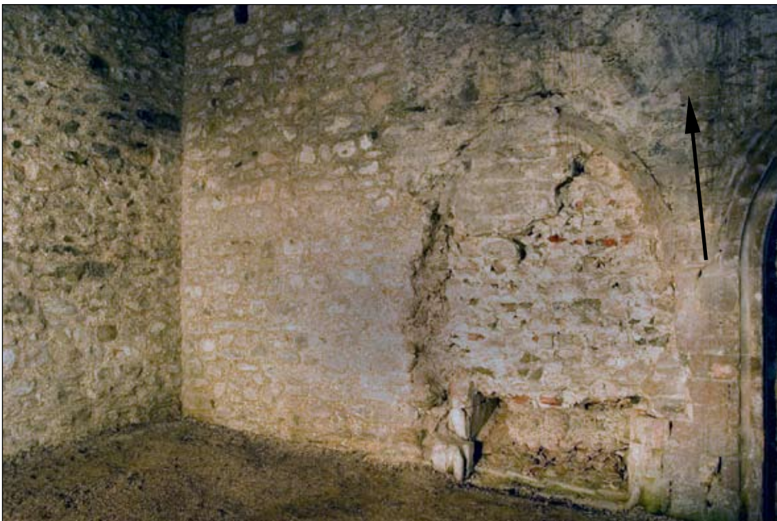
Figure 3. Line of voussoirs and stonework patch above service doorways
