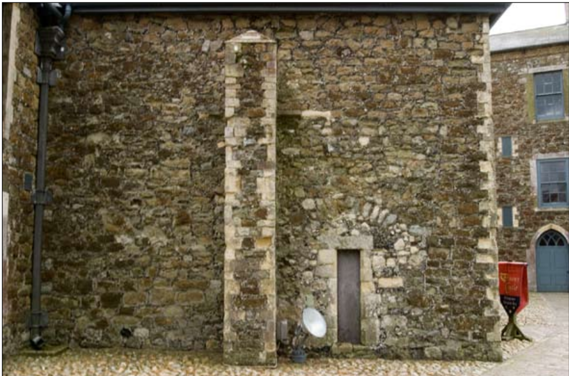
Figure 20. North-west wall of AV Building showing 'buttress' and remains of blocked arch between pentice and 'porch', now incorporated into the building
