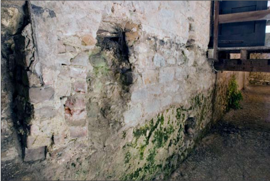
Figure 23. Layers of fabric from different phases, in the south-west wall of Arthur's Hall. Some 13th-century fabric at base (green), with three courses of possible 15th-century stonework above
