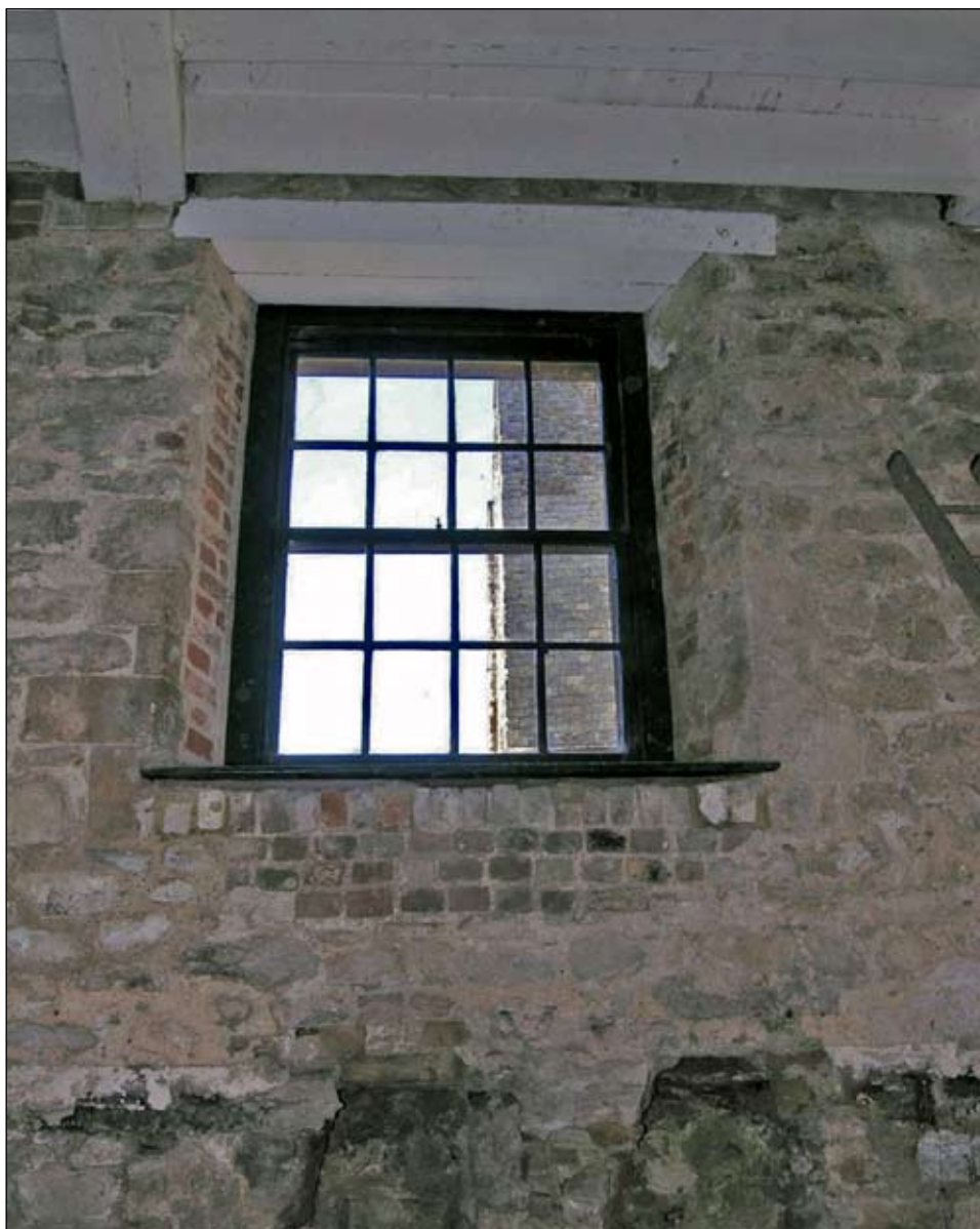
Figure 22. Sash window in Arthur's Hall showing surrounding patching where the window was inserted into a pre-existing wall
