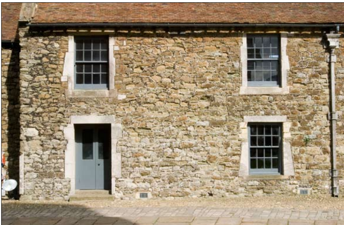
Figure 10. Joint between medieval rubble and regular 18th-century walling, to the left of the right-hand sashes
