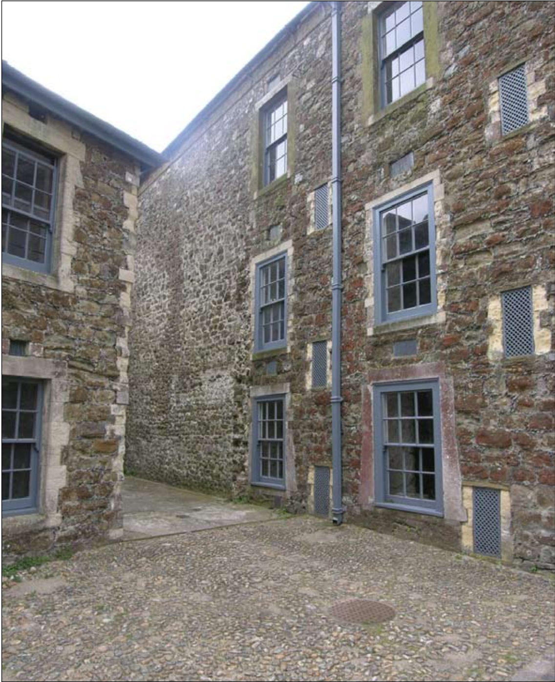
Figure 14. Keep Yard 7. External walling to right, with former internal fabric to the left
