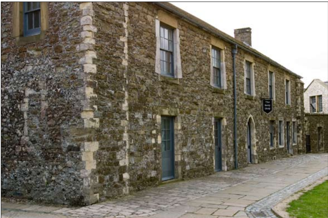
Figure 13. Arthur's Lesser Hall, now the shop. Rubble in the gable end and the lower walling of the façade contrasts with regular stonework at higher levels
