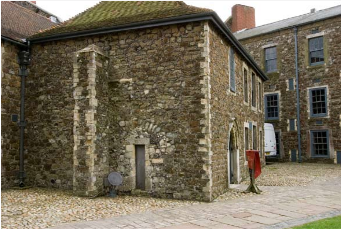
Figure 11. North-west wall of AV Building showing joint (at right side of end wall) between medieval rubble and regular 18th-century walling
