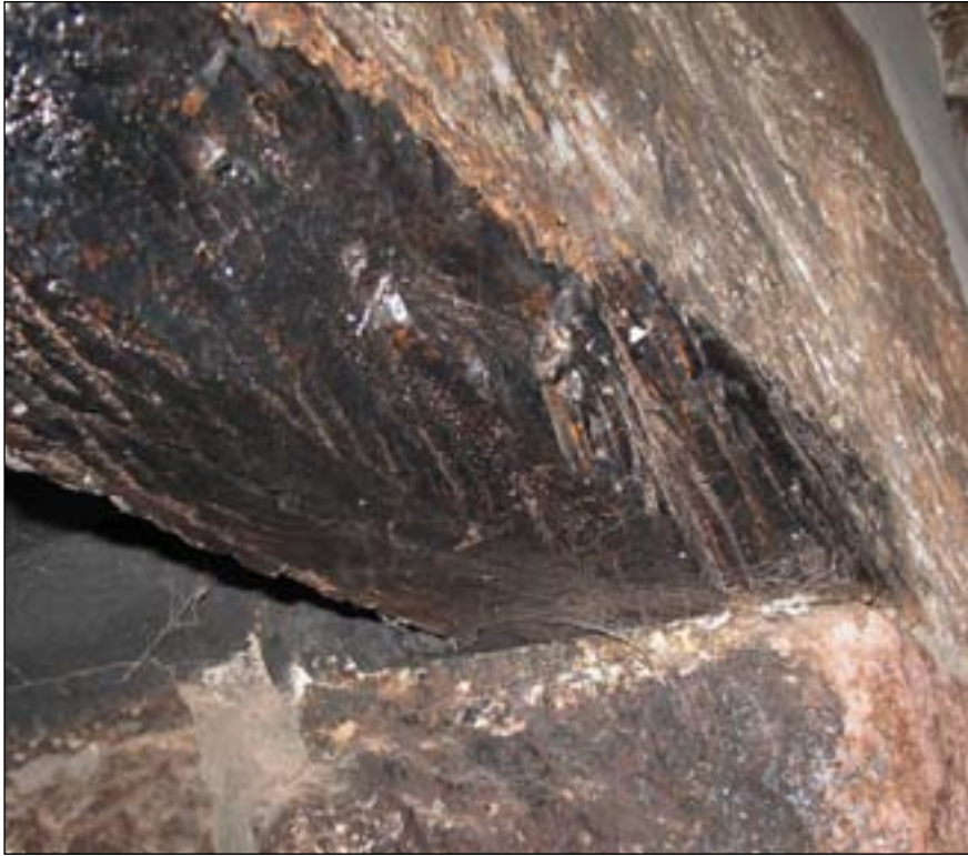
Figure 17. Detail of broach stop on bressumer of chimney breast at A-A1 (DPI13784).
