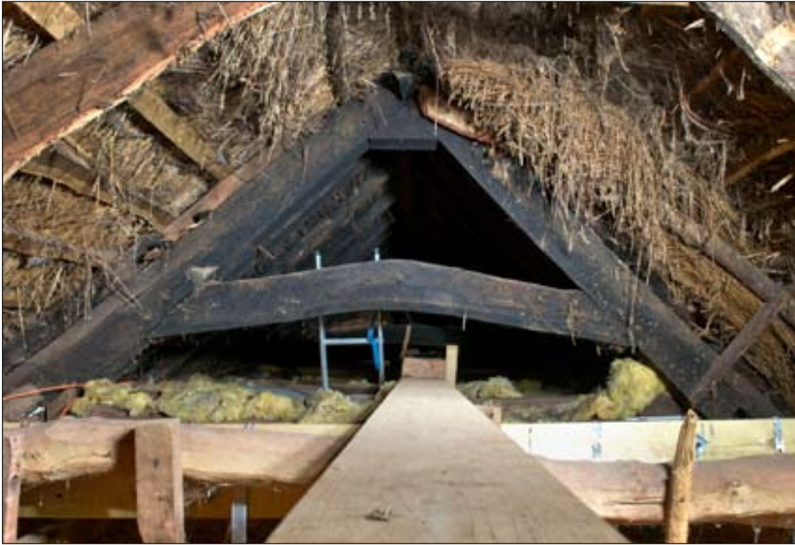
Figure 3. West face of cruck truss C-CI, also showing replaced timbers in Bay B-C (DPI13794).
