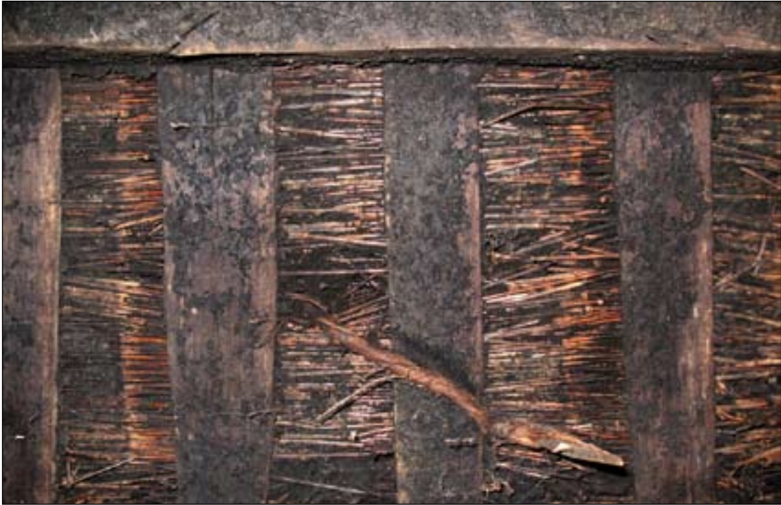
Figure 6. Detail of bay C-D, showing smoke-encrusted common rafters, laths, thatch and thatch ties (DPI13782).
