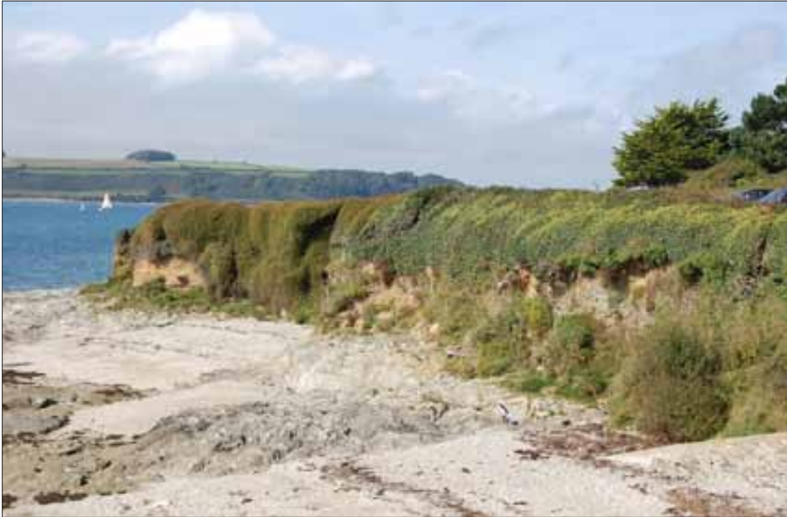
Figure 48. The cliff at Castle Cove, below the overflow car park to the north-west of St Mawes Castle, showing signs of erosion. Photograph by Abby Hunt.
