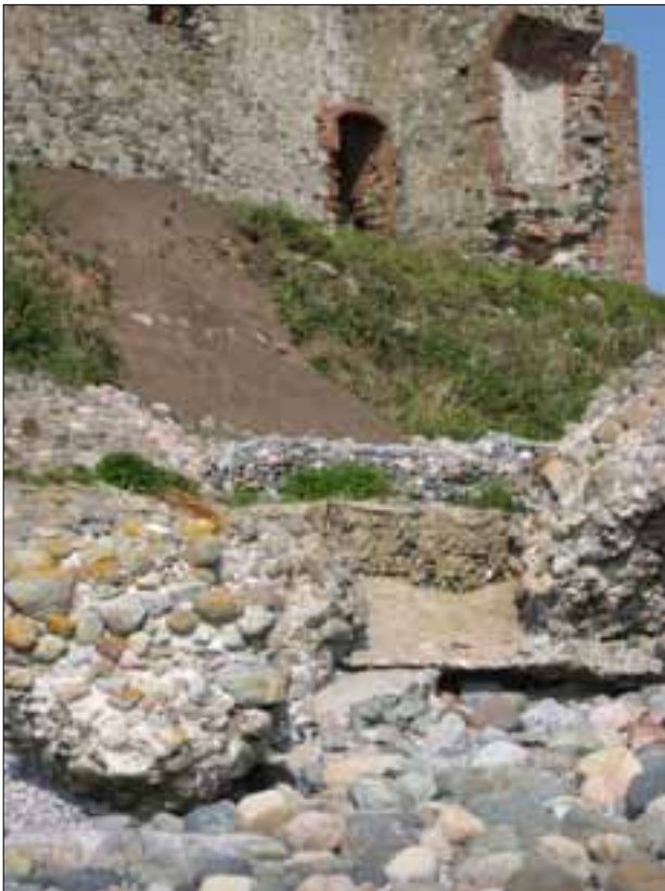
Figure 52. Erosion to the east of the keep. Photograph by Abby Hunt.
