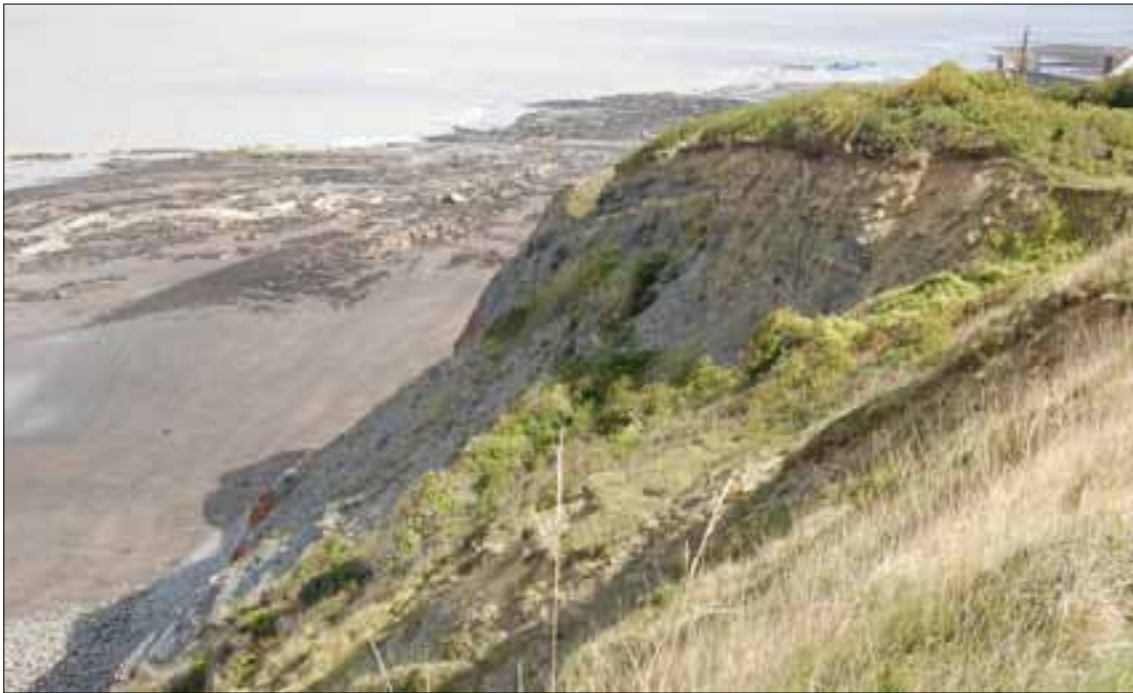
Figure 26. The cliffs immediately to the east of Daw's Castle; recent slippage visible in the photograph illustrate the friable nature of the rock. Photograph by Abby Hunt.
