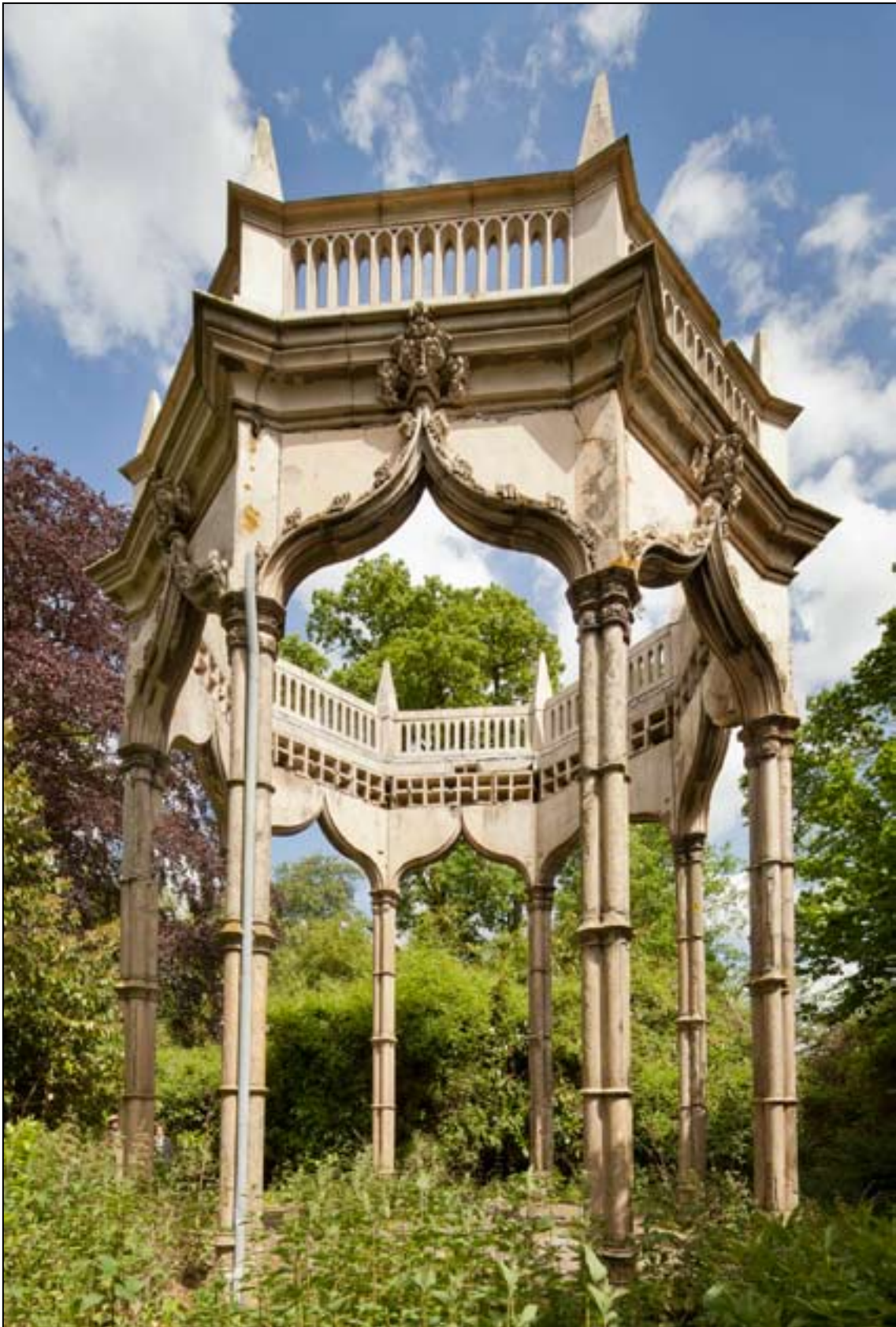
Figure 1. The 'Umbrello' has been neglected for many years and is now in imminent danger of collapse. Pat Payne DPI41279.jpg
