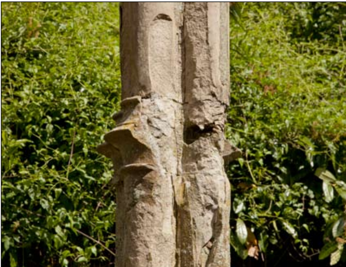
Figure 7. The 'Umbrello' showing one of the damaged clustered columns.
