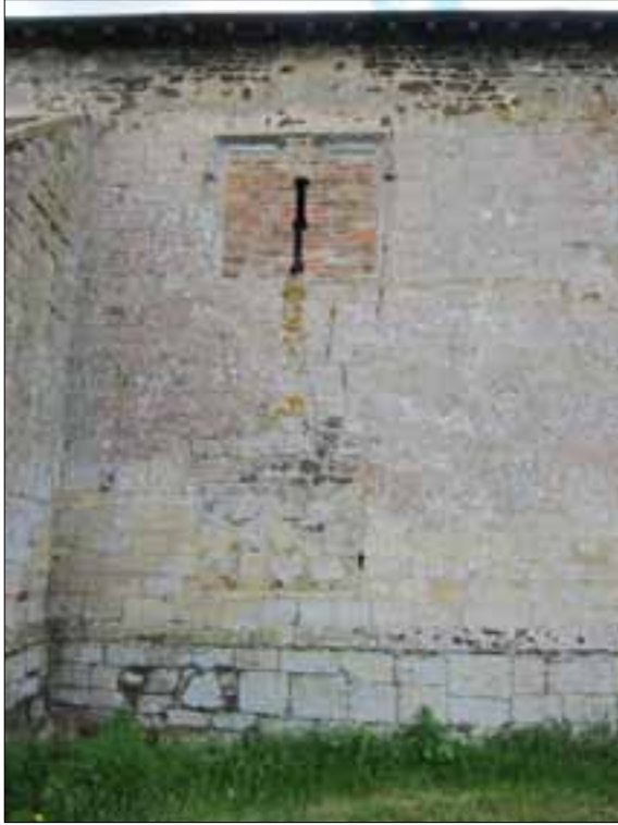
Figure 23. Blocked window at upper level with surviving hood mould on east façade.
