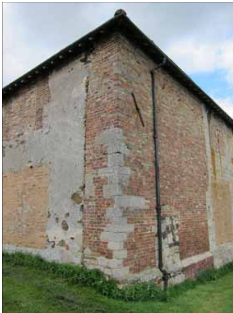
Figure 17. South-east corner, implying partial collapse and rebuilding.
