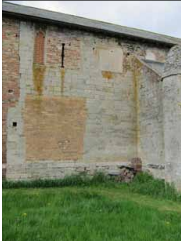
Figure 20. Blocked features, south façade.
