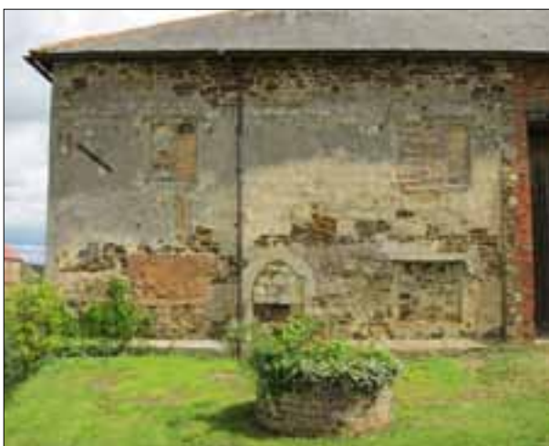
Figure 5. Blocked features on west façade.
