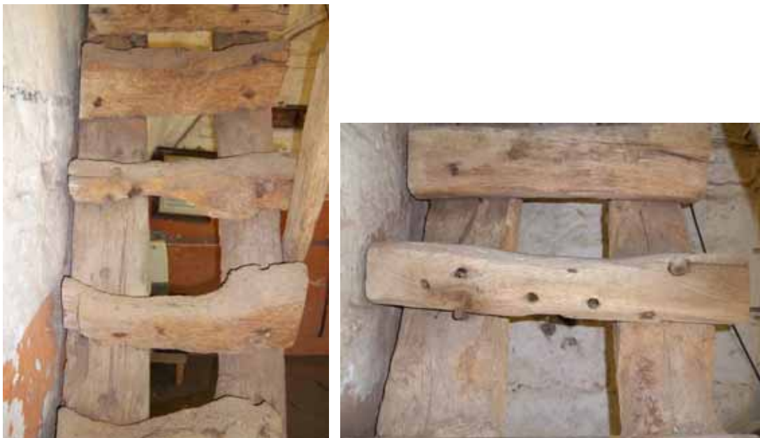
Figure 3c/d: Views of the ladder showing redundant mortice and peg holes in the wall stringer (left), and redundant peg holes in rung 11 (right)
