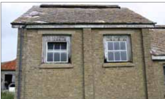
Figure 40. Detail of the taller part of later building, from the south-west or road side. The door is on the other side, facing the main workshop building.
