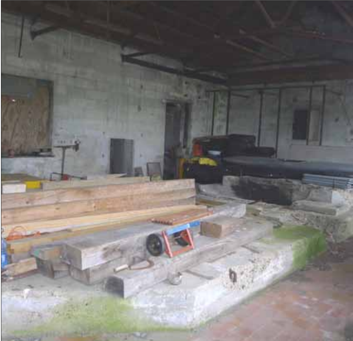
Figure 31. Interior of powerhouse.
