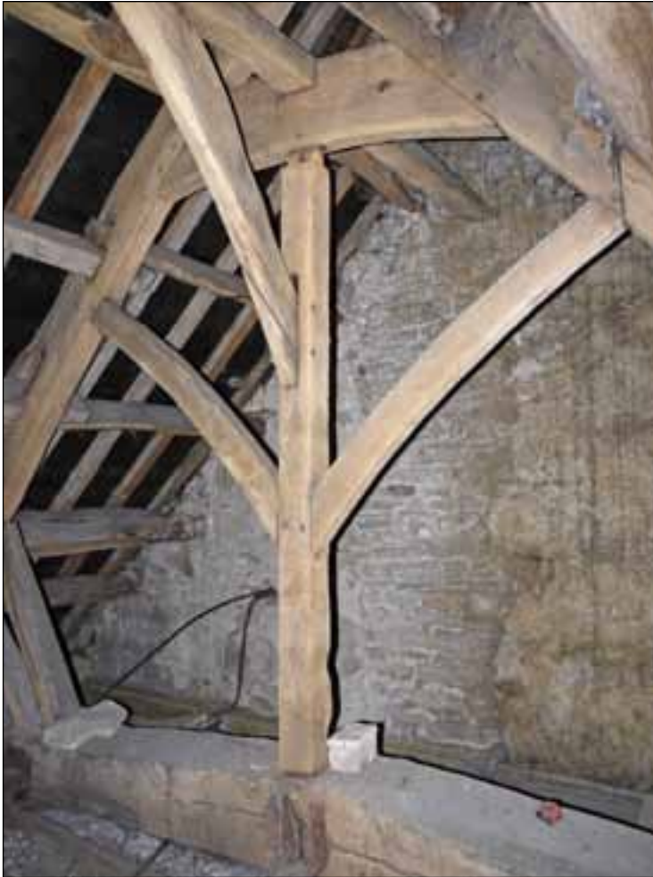
Figure 5. The hall's roof structure with inserted flue behind. (photograph: Adam Menuge, English Heritage).
