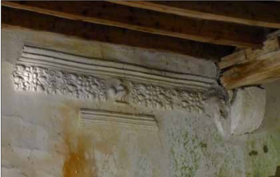
Figure 10. The decorative frieze on the first floor of the high-end tower (photograph: Adam Menuge, English Heritage).
