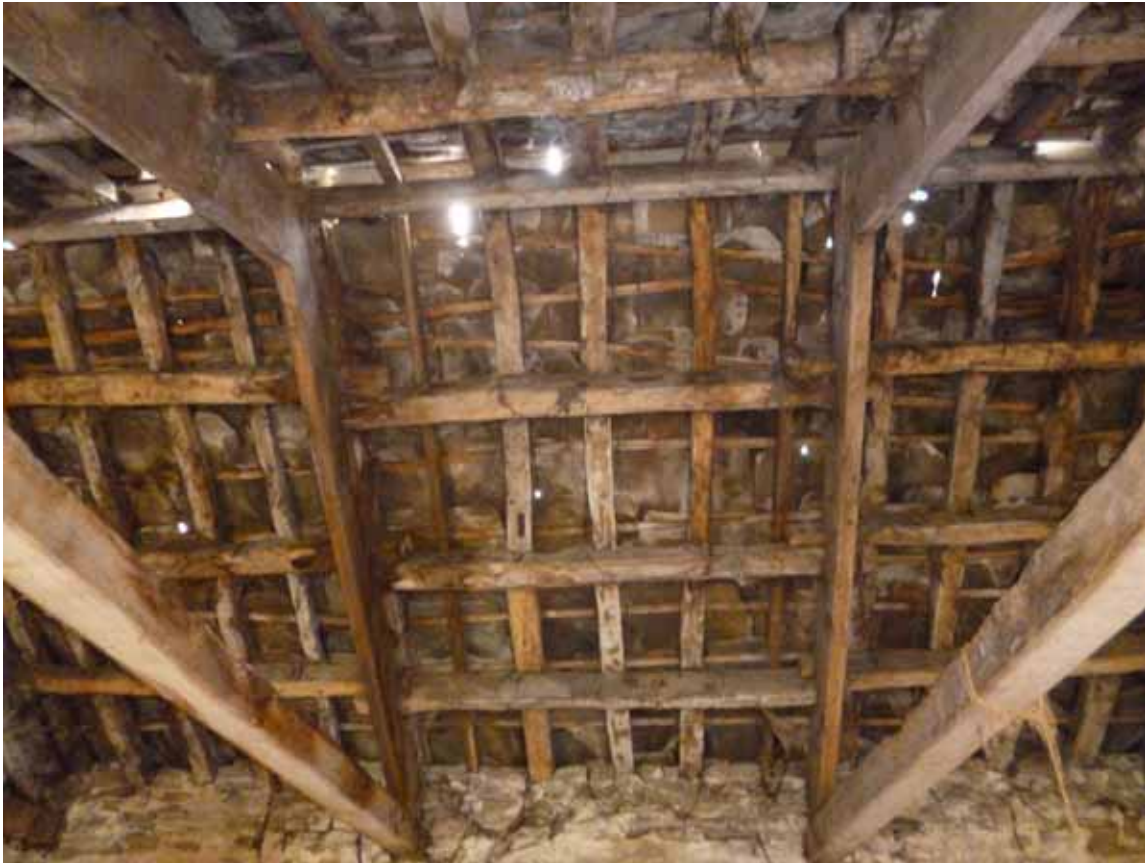
Figure 21: Stable/Coach-house range, stable roof, bay 7, photograph taken from the east (Robert Howard)
