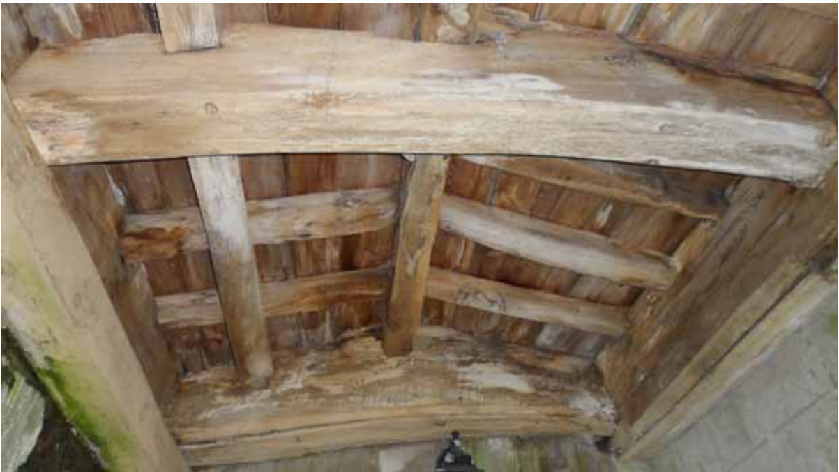
Figure 10: Porch roof, truss 2 in foreground, photograph taken from the south (Alison Arnold)
