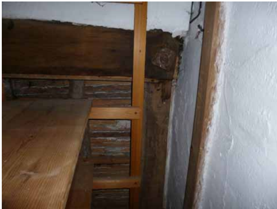
Figure 14: Service range, Kitchen roof, truss 1, photograph taken from the west (Alison Arnold)
