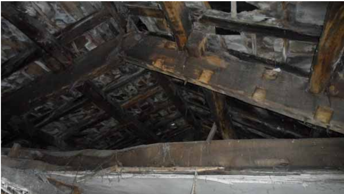
Figure 16: Service range, Tack room roof, truss 2, photograph taken from the west (Alison Arnold)
