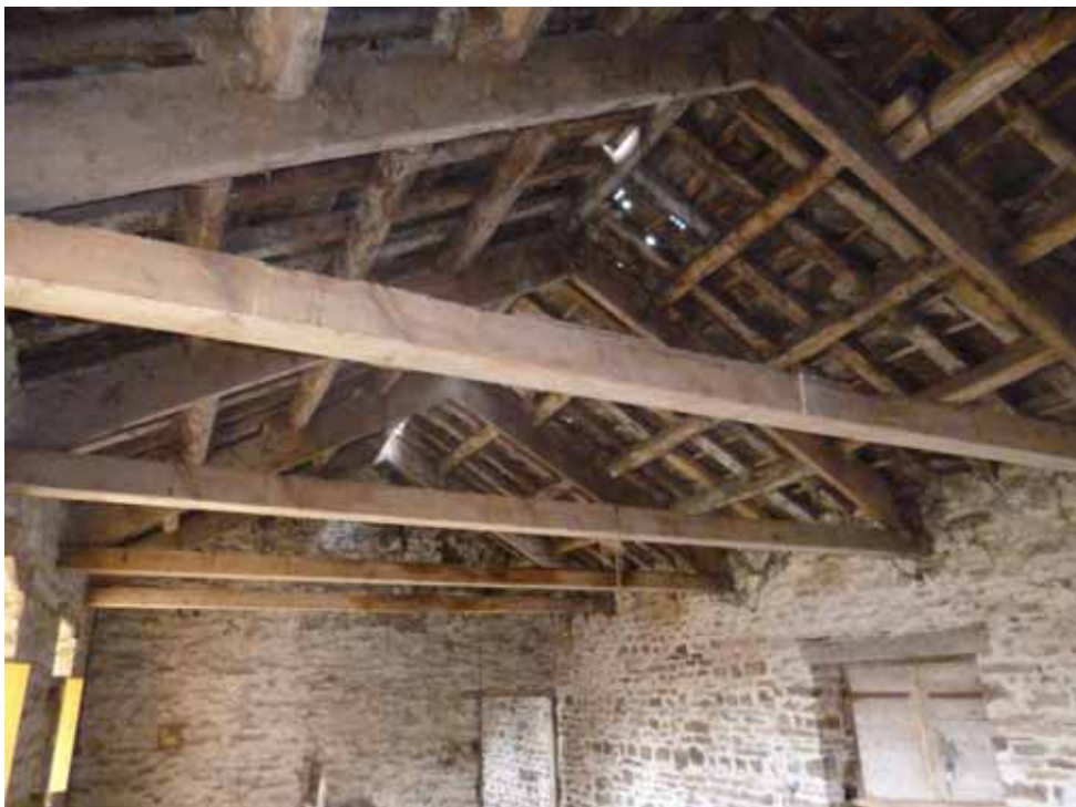
Figure 20: Stable/Coach-house range, stable roof, truss 6 in the foreground, photograph taken from the north (Robert Howard)
