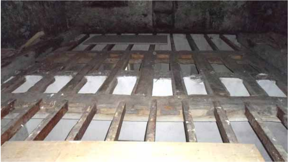
Figure 7: High-end tower, first-floor ceiling frame (from above) with main beams from the second floor lain loose by the walls (Alison Arnold)
