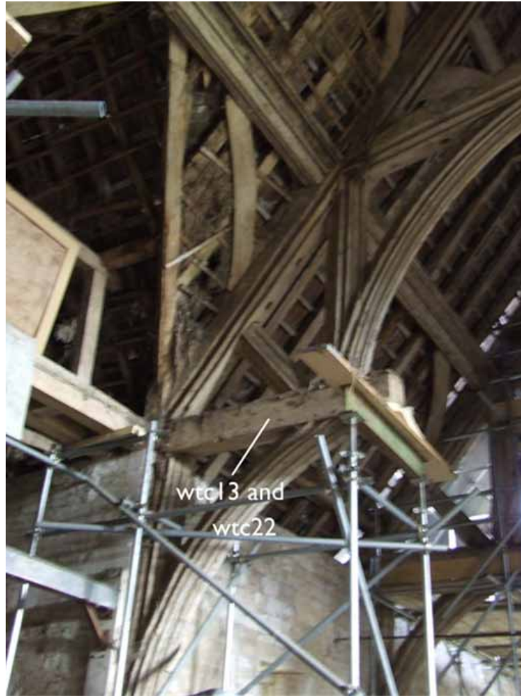
Figure 7: Photograph, looking north-east, showing the north-west side of truss 4, with the hammer beam sampled twice indicated (Martin Bridge)
