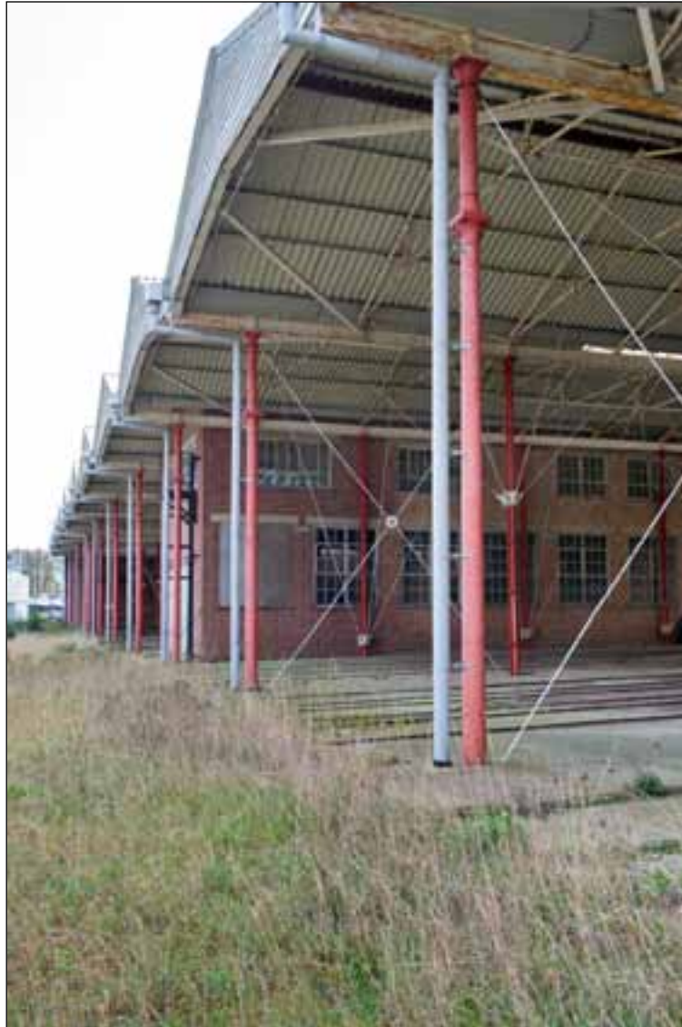
Figure 38. Columns at front of gunboat shed cast in two pieces and joined together. Ordinary cross-sectioned columns are visible behind these. (EHA DPI61538)
