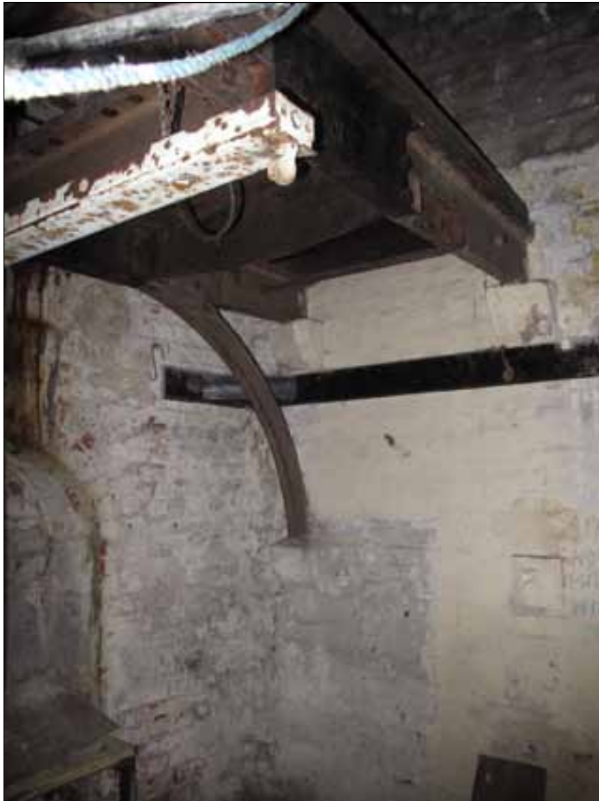
Figure 52. Interior of rebuilt well house showing part of winch mechanism (© English Heritage)
