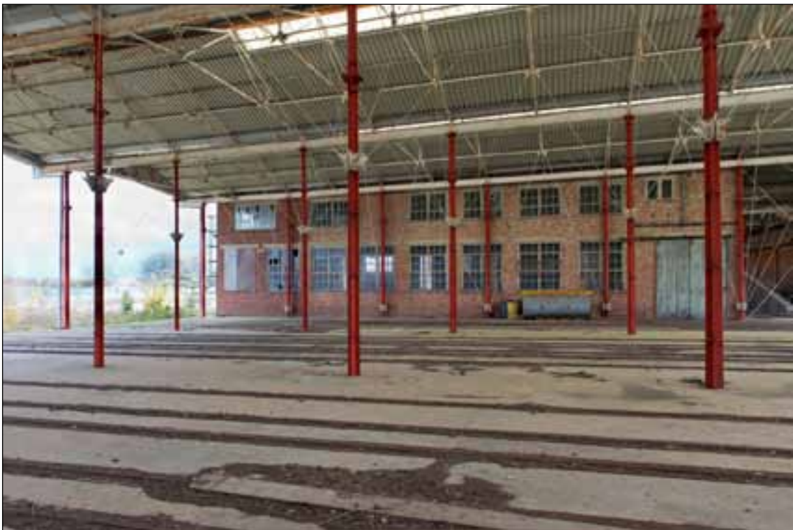
Figure 34. Interior of gunboat sheds showing the west elevation of the inserted brick building (EHA DPI61558)
