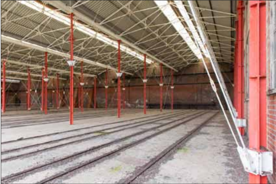
Figure 35. Gunboat shed interior from north west, showing the three sets of rails present in the standard bays (EHA DPI61544)
