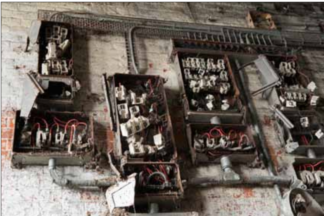
Figure 51. Fuseboxes on the west wall of the boiler house (EHA DPI61563)
