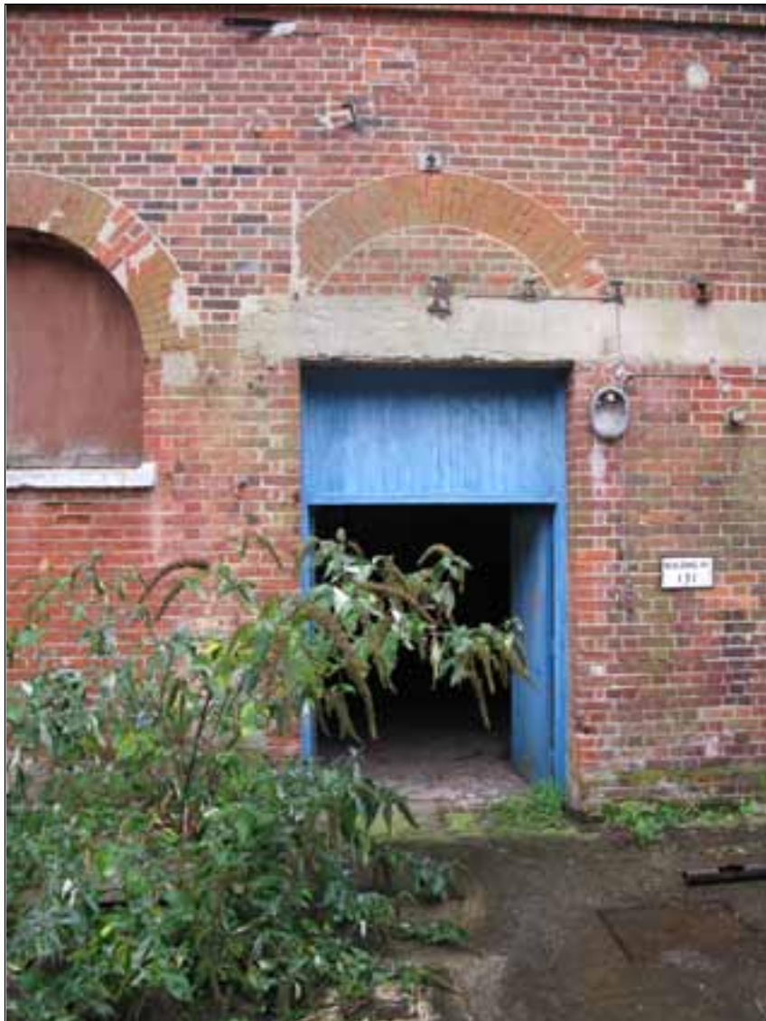
Figure 45. North elevation of the boiler house showing the inserted doorway (© English Heritage)
