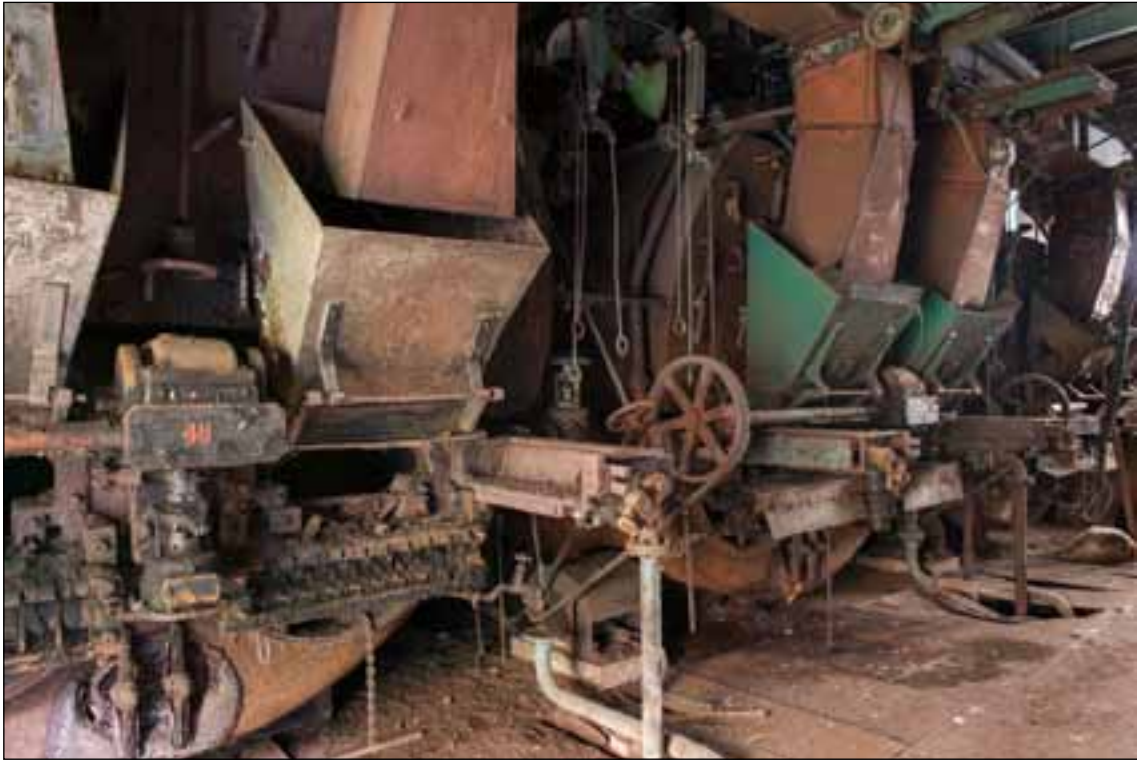
Figure 50. Lancashire boilers, with a later automated hopper system (EHA DPI61559)
