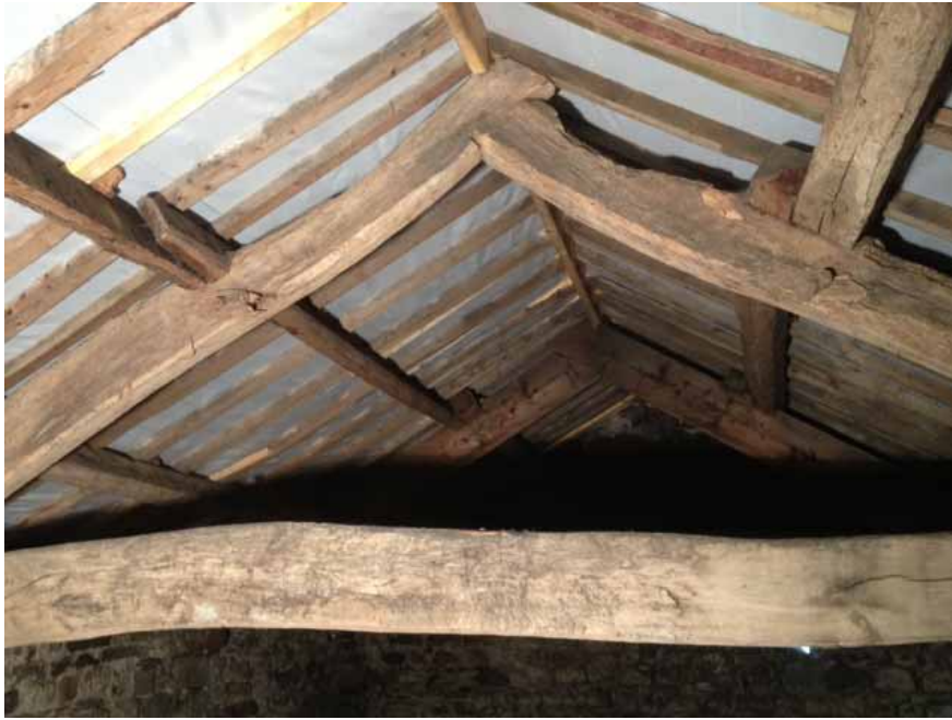
Figure 5: The roof, with truss 2 in the foreground, photograph taken from the west (Alison Arnold)
