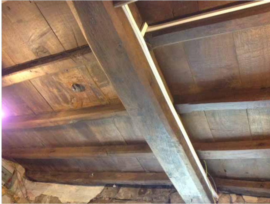
Figure 7: First-floor frame, viewed from below in the kitchen, photograph taken from the north-west (Alison Arnold)
