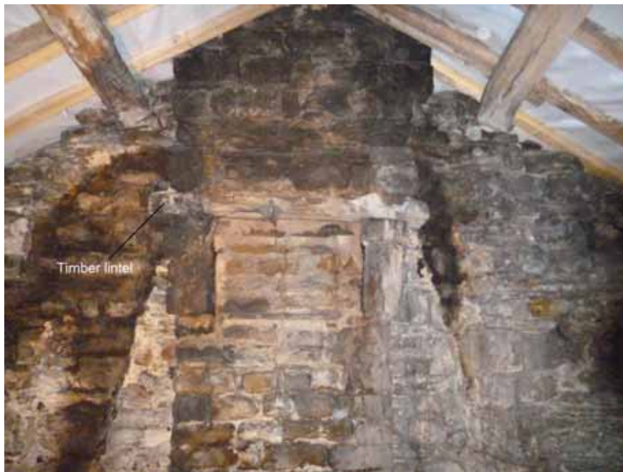
Figure 6: Chimney stack with timber lintel, photograph taken from the east (Alison Arnold)
