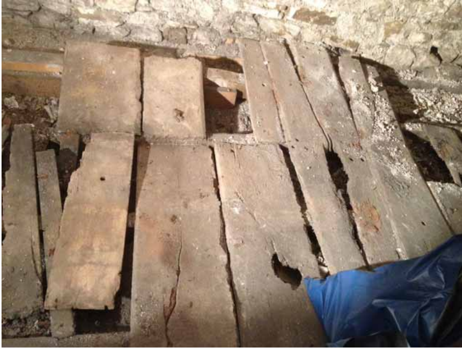
Figure 9: Attic floorboards, some of which can be seen to have peg holes (Alison Arnold)
