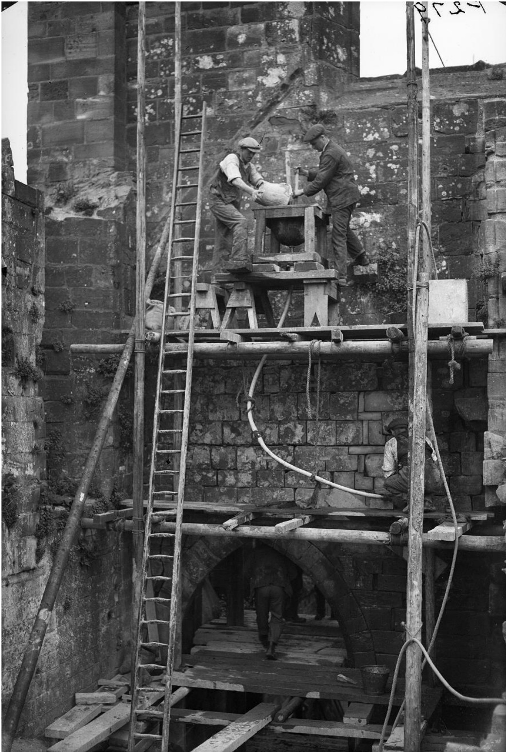
Figure 27: The gravity grouting machine being used to repair the walls at Furness Abbey, Cumbria, in the 1920s. Copyright English Heritage.
