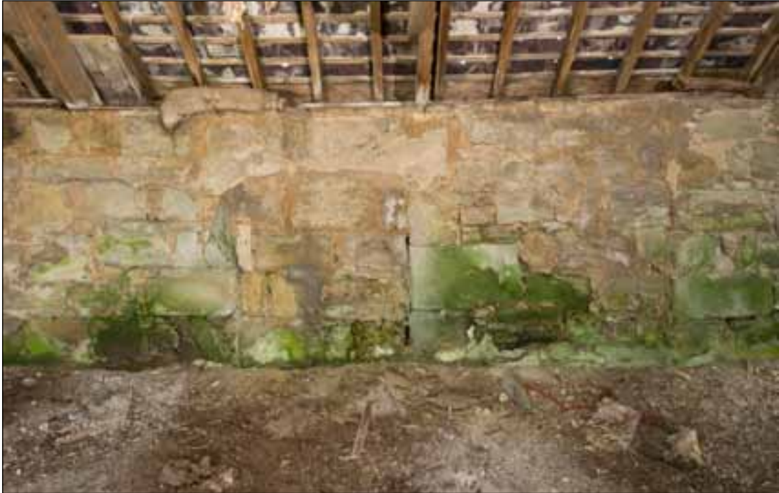
Figure 15: The south-west wall at first-floor level showing internal straight joints and blocking (DPI56959 © English Heritage, photograph: Alun Bull).
