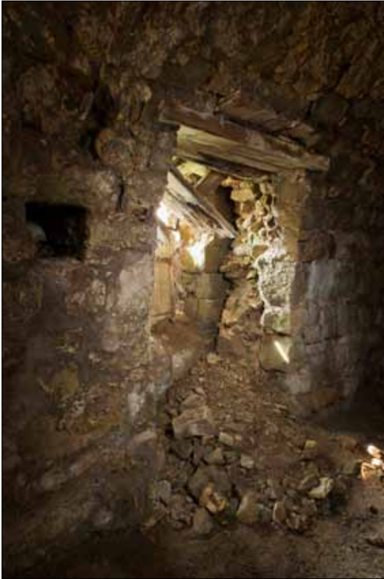
Figure 14: The dressed-stone wall face revealed behind the collapsed soffit and jamb of the opening in the centre of the south-west wall (DPI56931 © English Heritage, photograph: Alun Bull).
