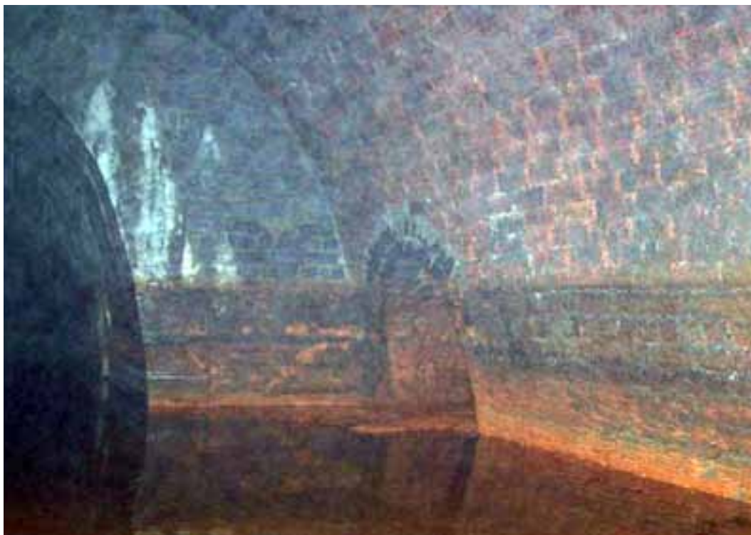
Figure 14: Remaining open entrance to Carr Pit wagonway, seen in south wall of tunnel, just west of narrowed section of the wide hole, looking south-east (after Cordon 2006, image 79), © Tina Cordon, reproduced with permissions
