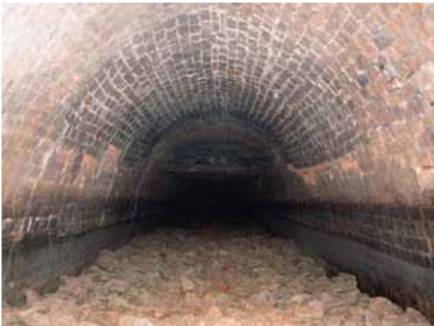
Figure 7: Limestone infill in the Butterley Tunnel, (after Witter 1979, image 13) © Robin Witter, reproduced with permissions
