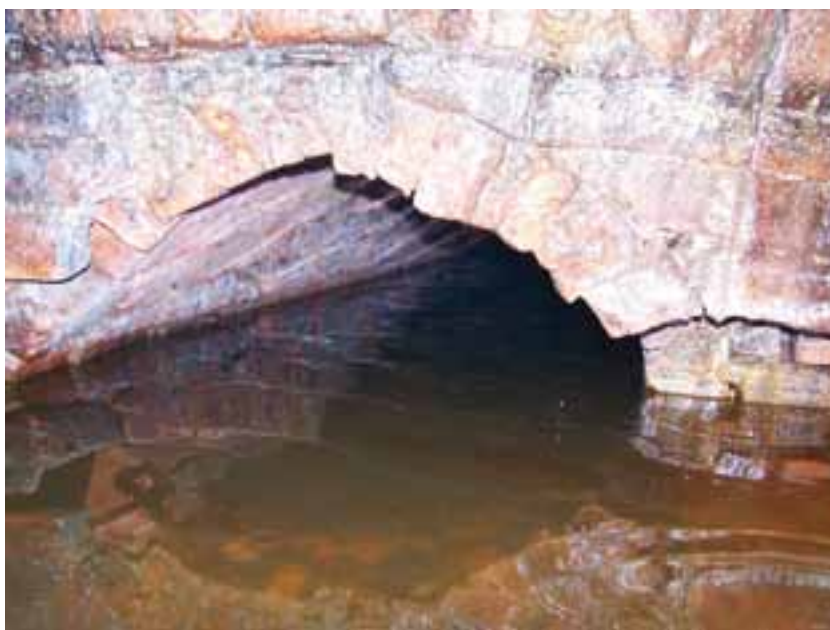
Figure 12: Low entrance to blast receiver passage in north wall of tunnel, looking north (after Cordon 2006, image 59), © Tina Cordon, reproduced with permissions
