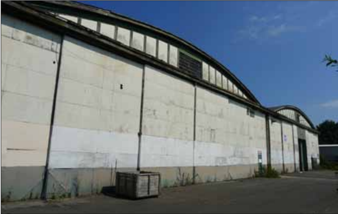
Figure 12: Sliding doors at the south-east end of Building 18 (© English Heritage, photograph: Clare Howard).
