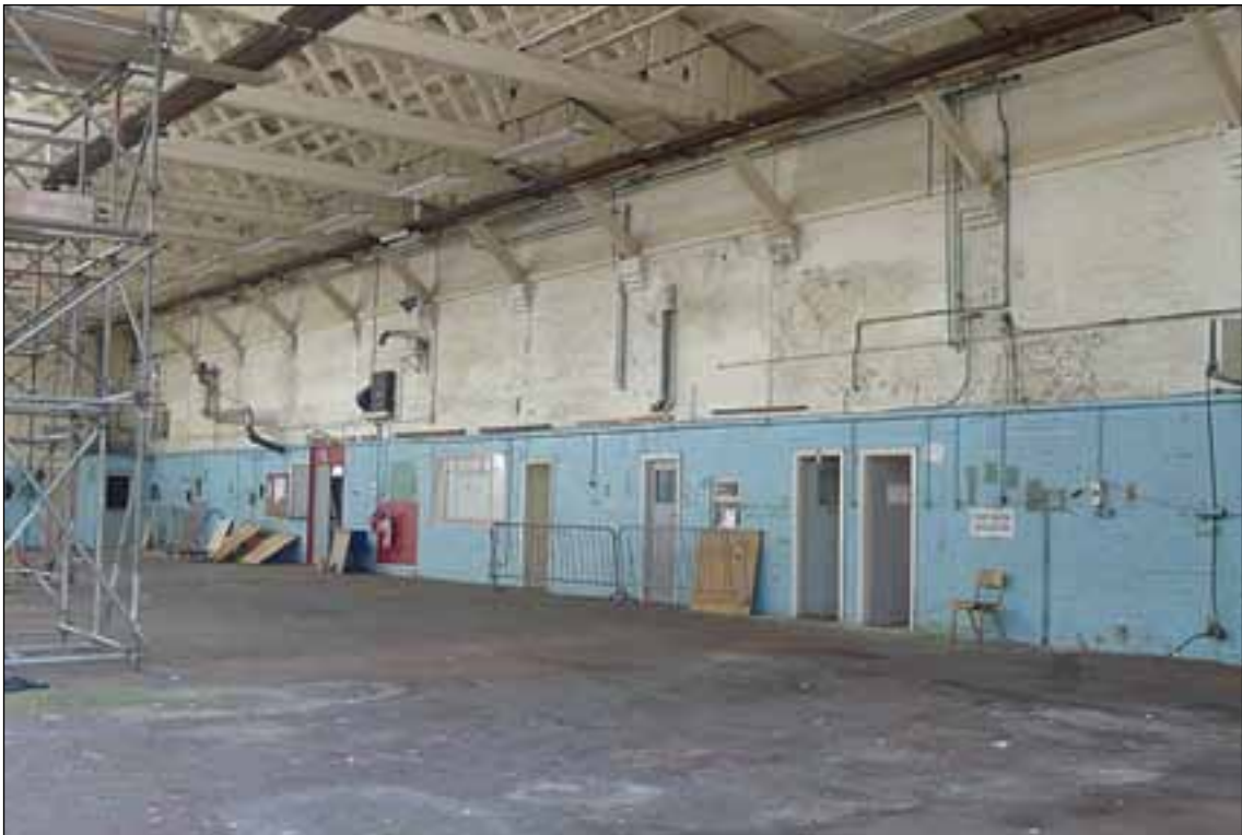
Figure 21: Interior of Building 18 showing the blocked arches (© English Heritage, photograph: Clare Howard).
