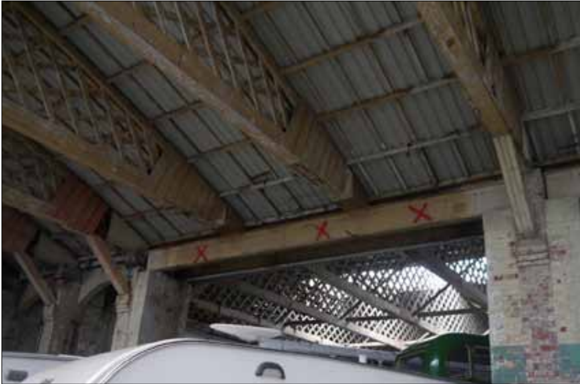
Figure 24: Central arcade showing where the arches have been removed and replaced by an RSJ, Building 17 (© English Heritage, photograph: Simon Taylor).
