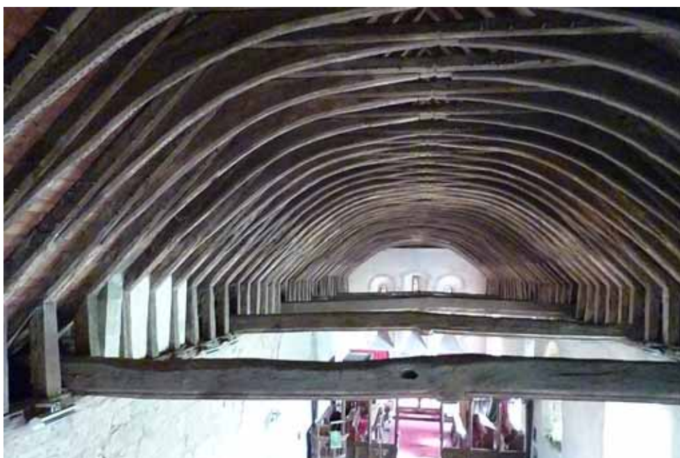
Figure 3: View of the nave roof looking west to east (photograph Robert Howard)
