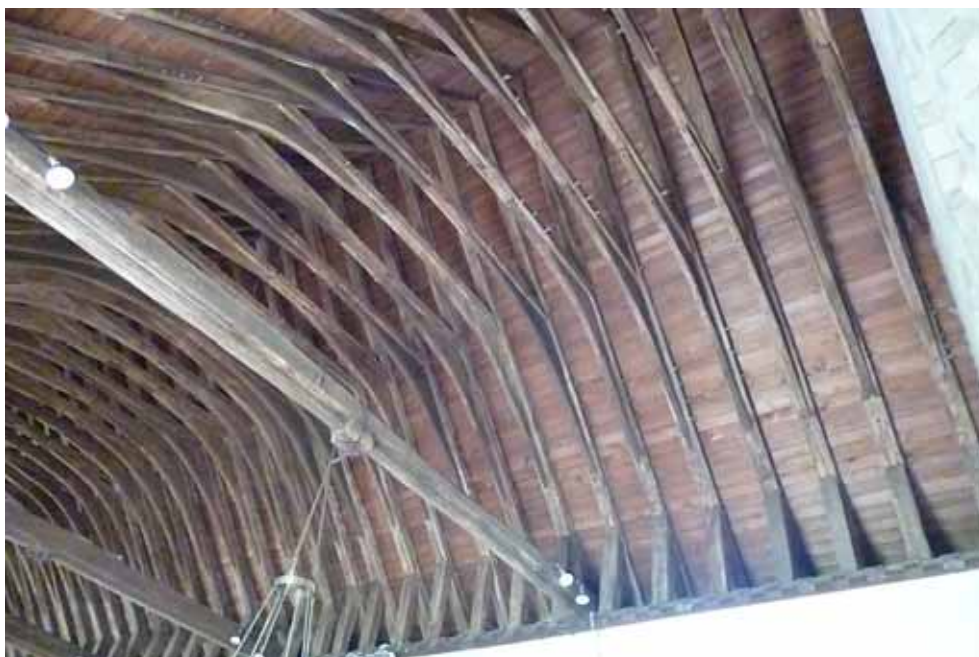
Figure 2: View of the chancel roof of St Mary's Church (photograph Robert Howard)
