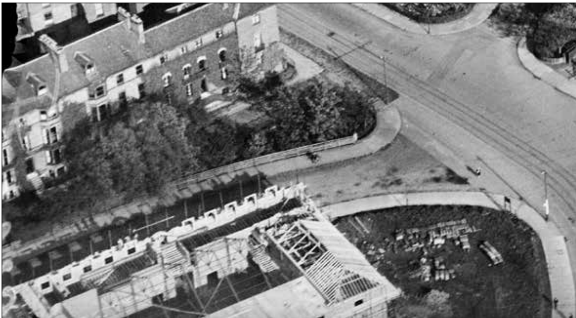
Fig 81 Tynemouth's drill hall is seen under construction in an aerial photograph taken in October 1927. © English Heritage EPW019755
