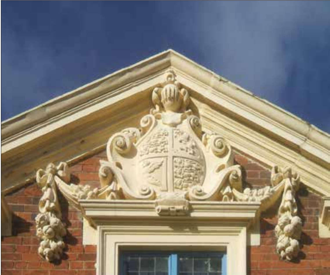
Fig 53 The cartouche and crest of Bilston's drill hall, unusually elaborate details for such a modest sized building. © John M. This work is licensed under the Creative Commons Attribution-Share Alike 2.0 Generic Licence
