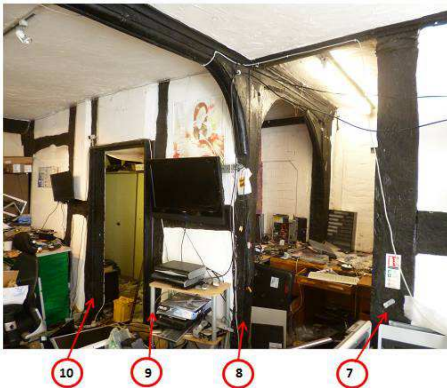
Figure 4a/b: Views to help locate sampled roof (top) and ground-floor timbers (bottom) (photographs Robert Howard)
