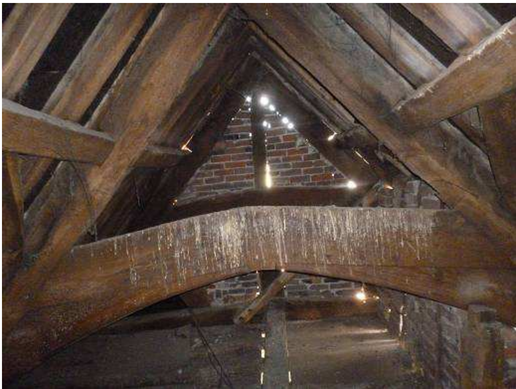
Figure 2a/b: Views of the impressive timber framing to the first floor (top) and the inaccessible trusses (bottom) (photographs Robert Howard)
