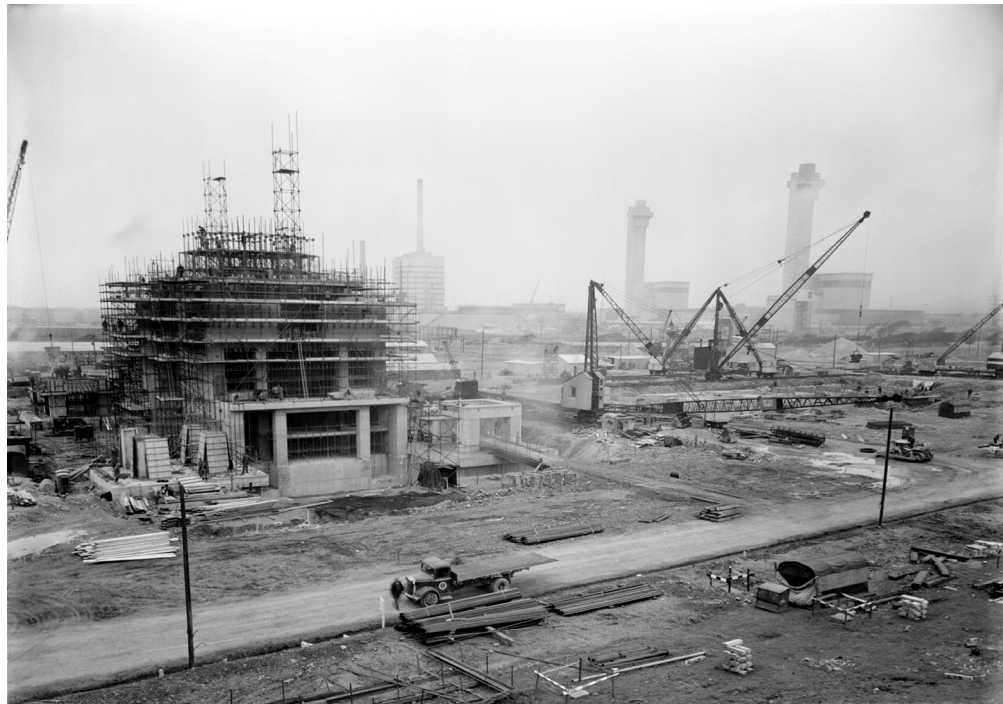
Figure 8 Windscale, Calder Bridge (later Calder Hall) Cumbria, April 1954, work underway on the PIPPA reactors, to the right are the Windscale Piles © Crown copyright.NMR G5074-3
